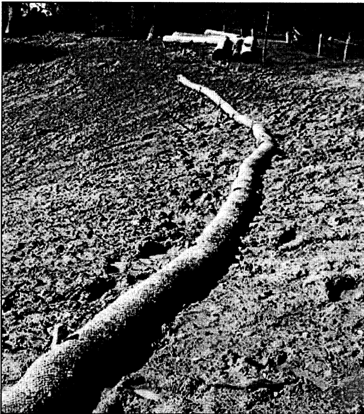
Left: Fiber rolls at Greens Complex 18 not properly staked. Improperly installed fiber rolls are not effective in filtering runoff or slowing it down.
