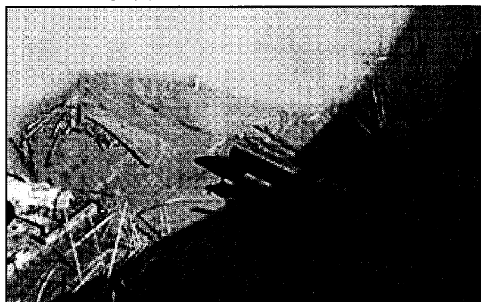
Below: Some construction areas drain to pond. Photo shows muddy water in pond and accumulated sediment below drainage pipe.
