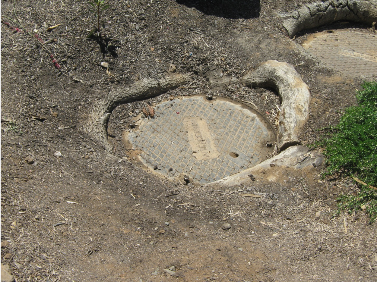
Grease Trap Access Upper Parking Lot
