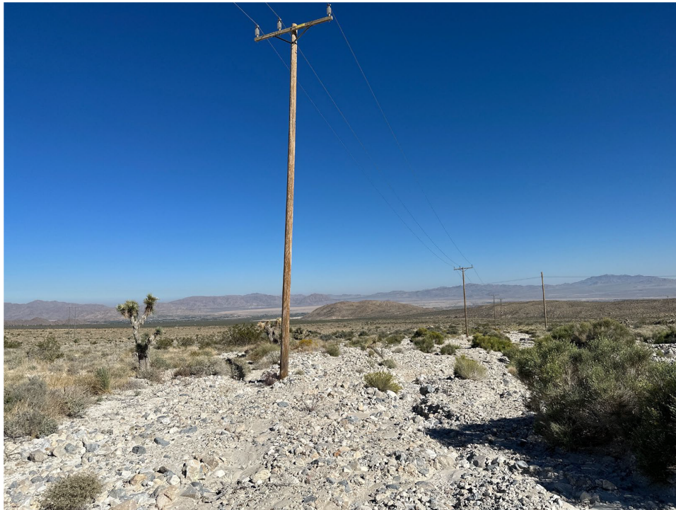
Photo 3. Pole 1738226E, View Facing North
