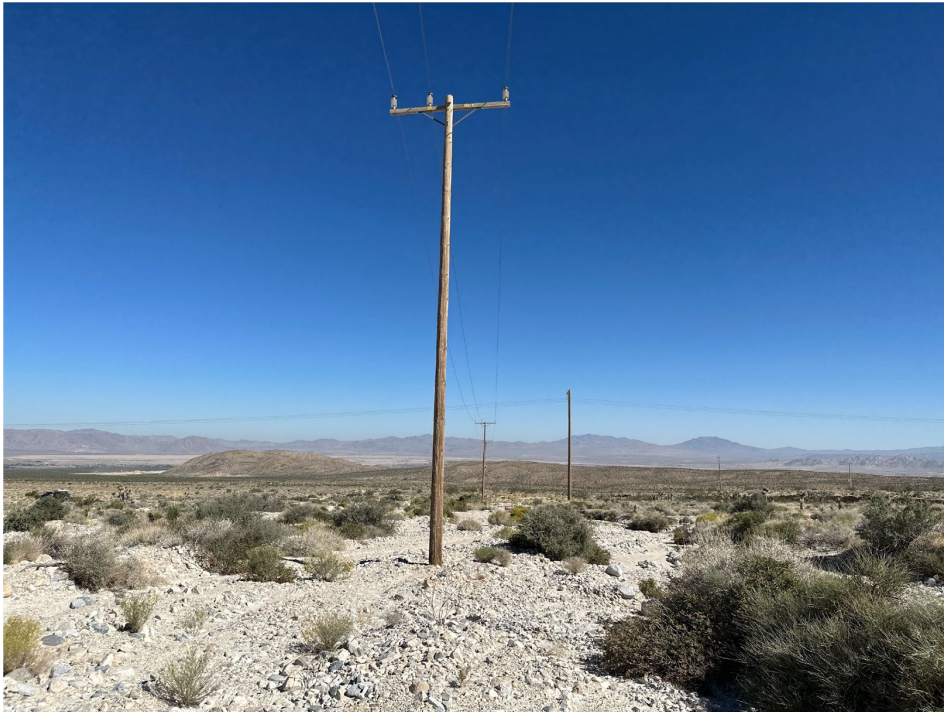
Photo 2. Pole 1738227E, View Facing North
