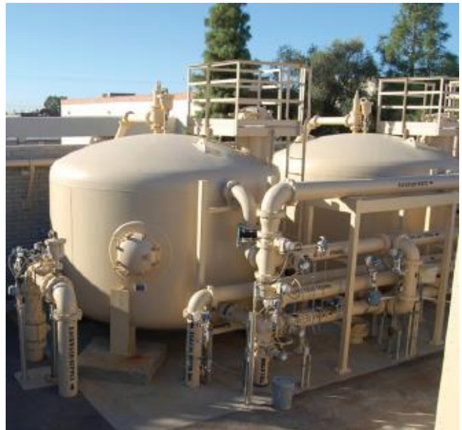
Figure 1. Keyes CSD Arsenic Treatment Plant
