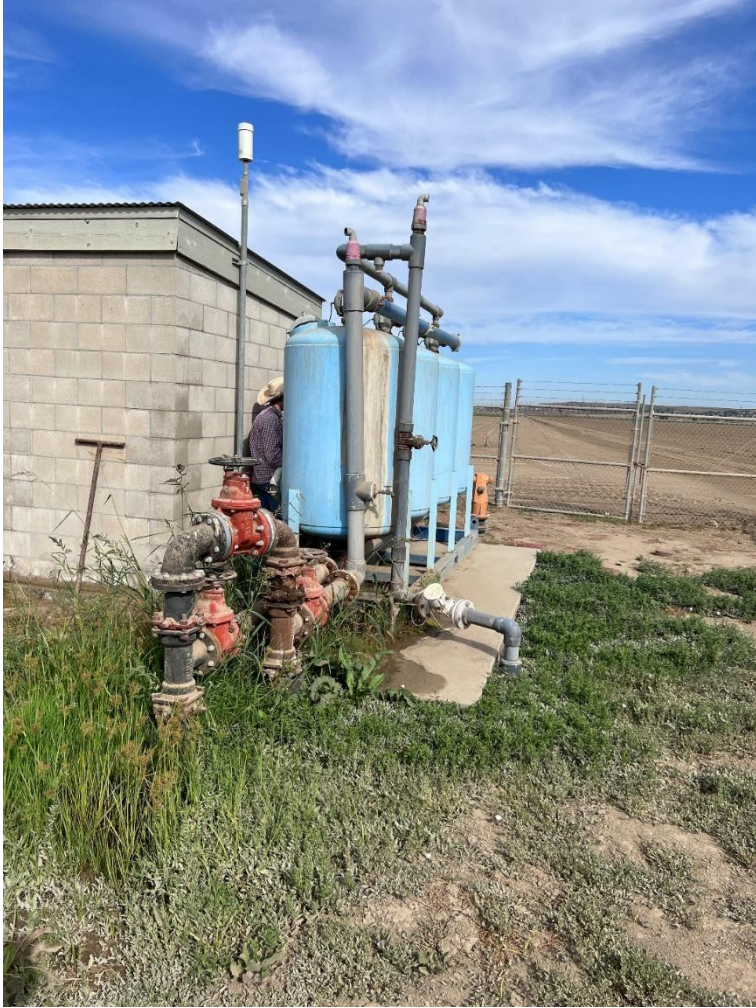
Manganese Dioxide Filtration System
