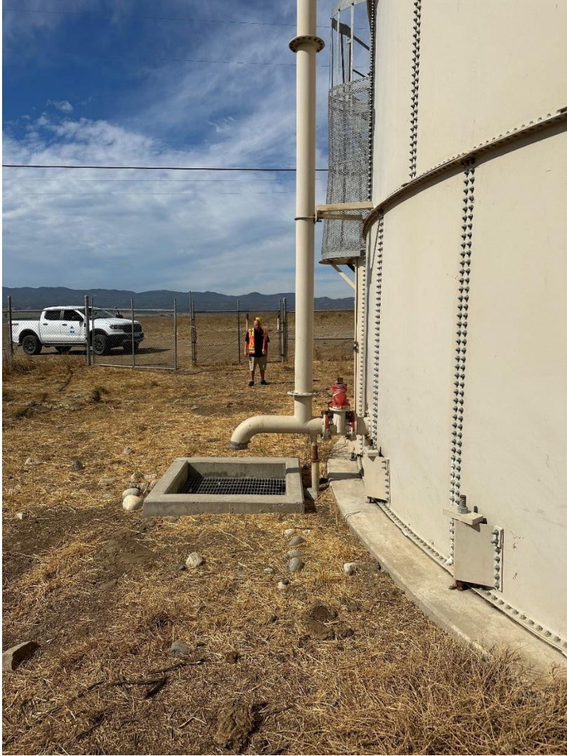
Overflow Drain and Piping
