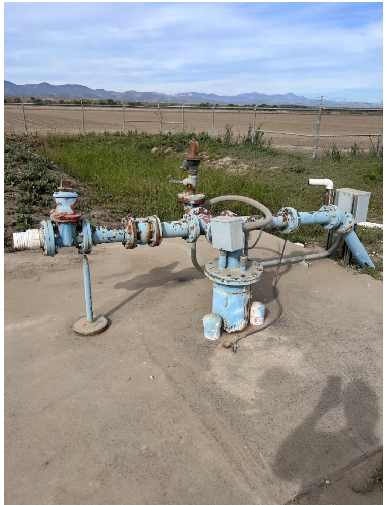
Abandoned Well #2 at Treatment Facility
