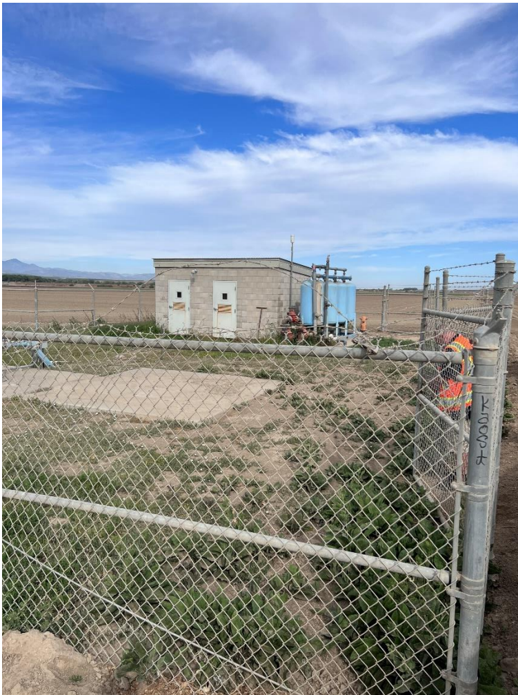
Water Treatment Facility Overview
