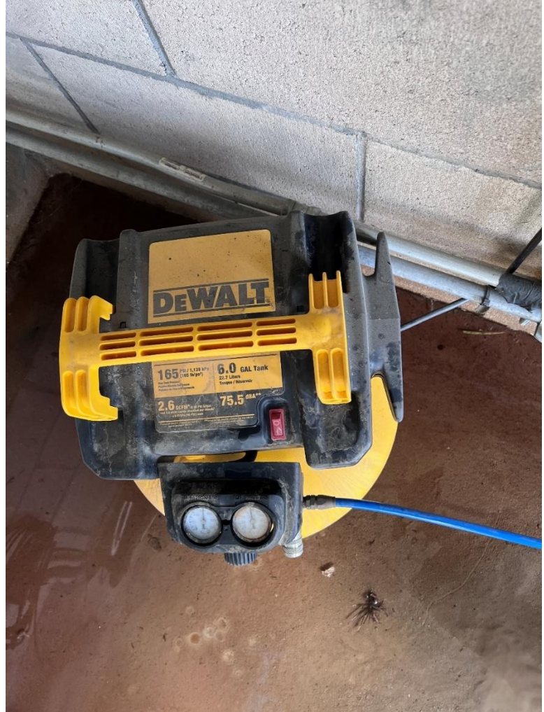
Treatment Facility Air Compressor
