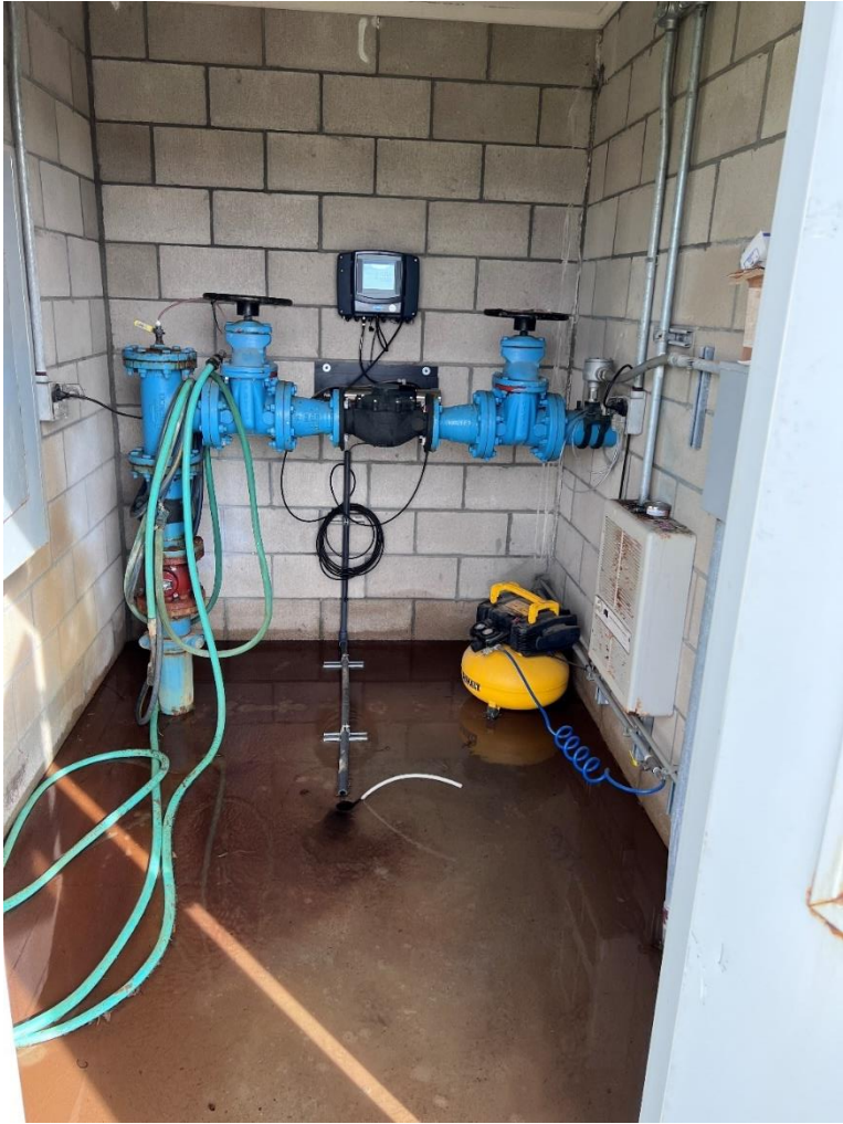
Sodium Hypochlorite Injection Facilities
