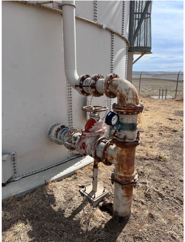
Storage Tank Inlet/Outlet
