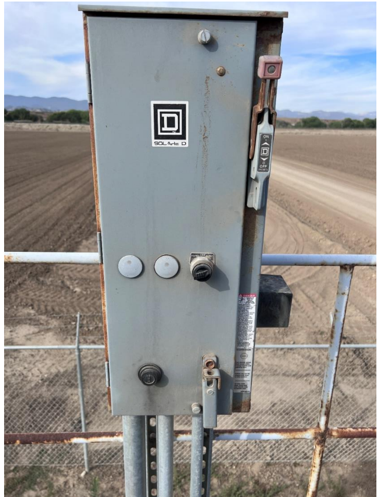
Well #3 Electric Control Panel
