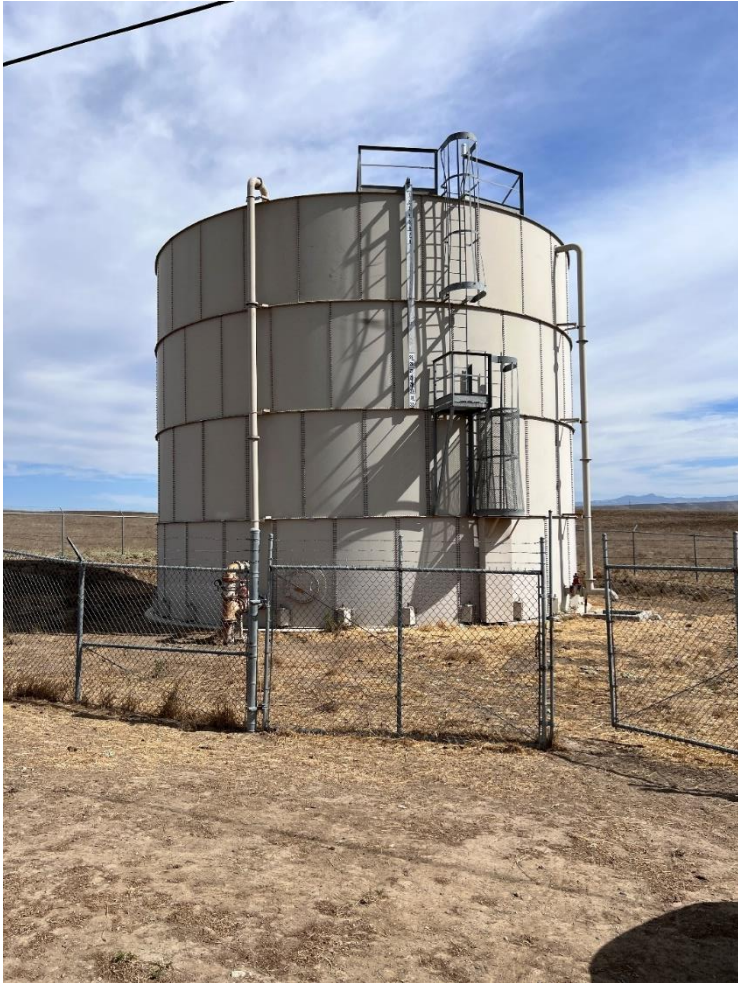
Overview of Storage Tank
