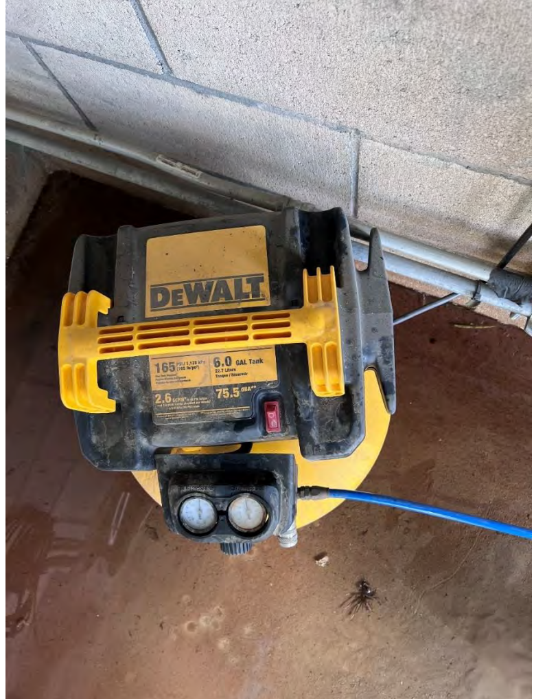
Treatment Facility Air Compressor
