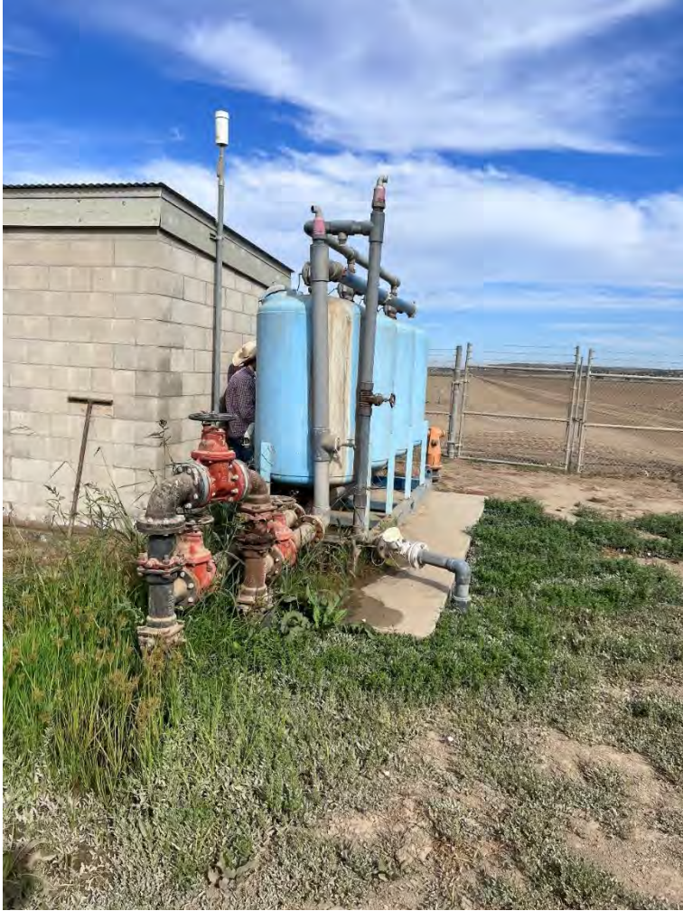
Manganese Dioxide Filtration System
