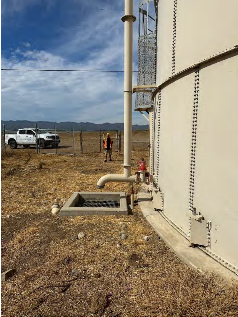
Overflow Drain and Piping
