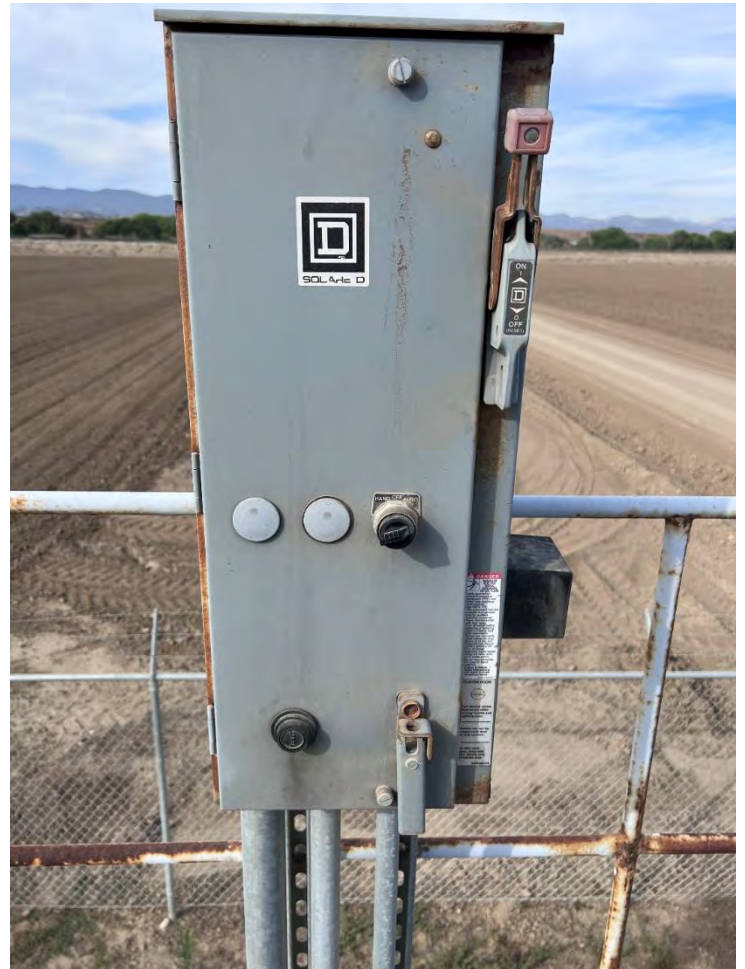
Well #3 Electric Control Panel
