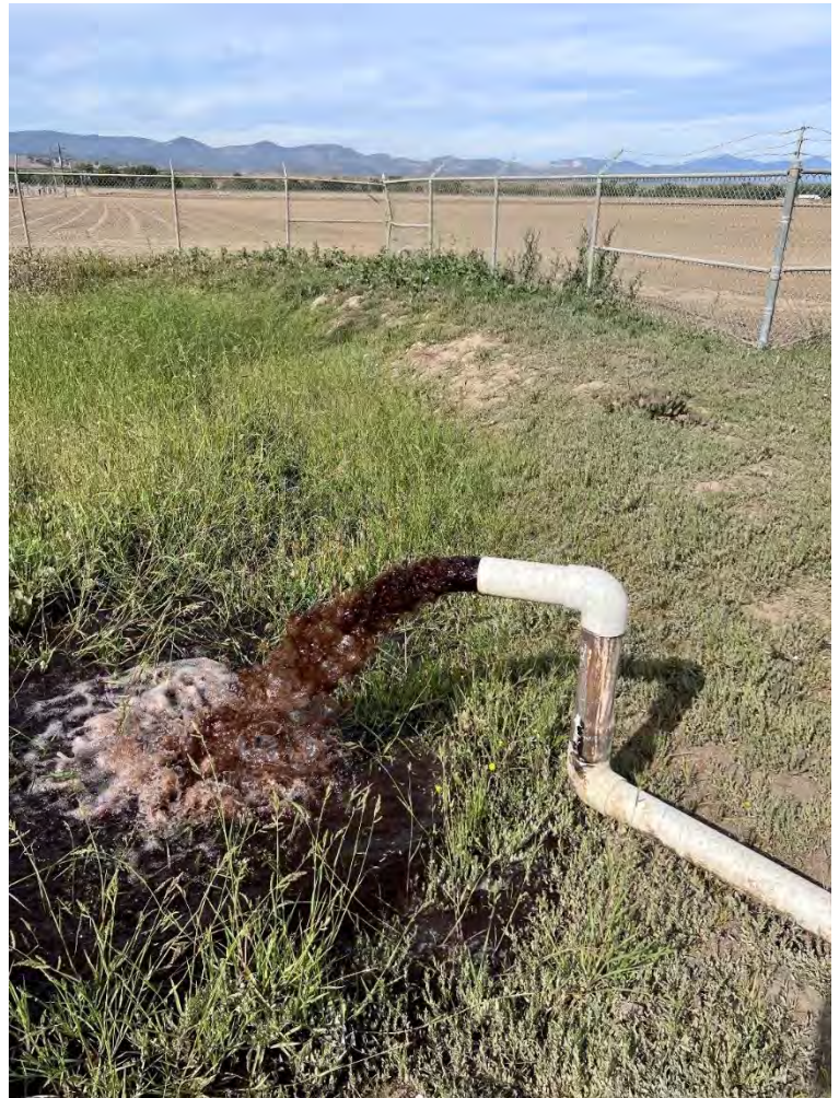
Wastewater from Filter Backwash
