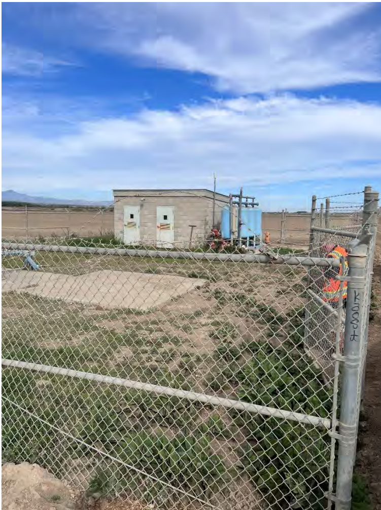
Water Treatment Facility Overview
