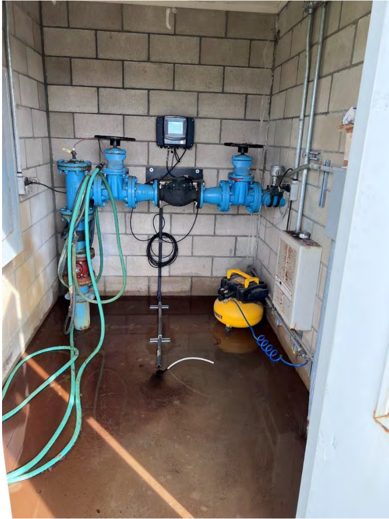
Sodium Hypochlorite Injection Facilities
