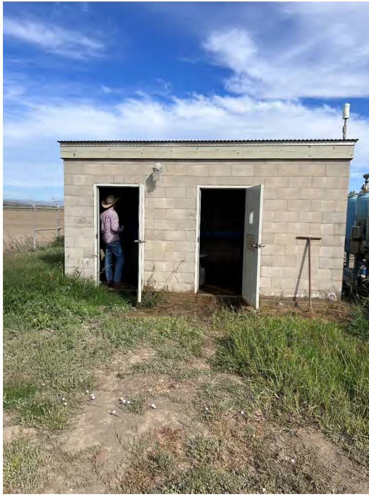
Chemical Storage/Injection Building
