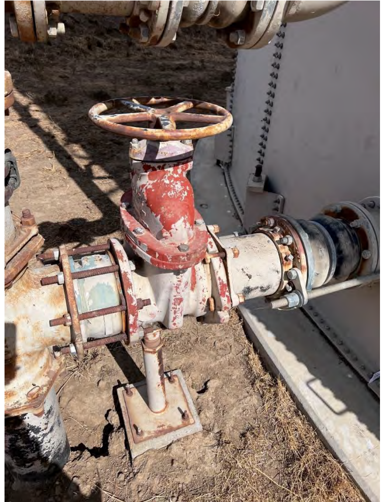
Outlet Flow Control Valve
