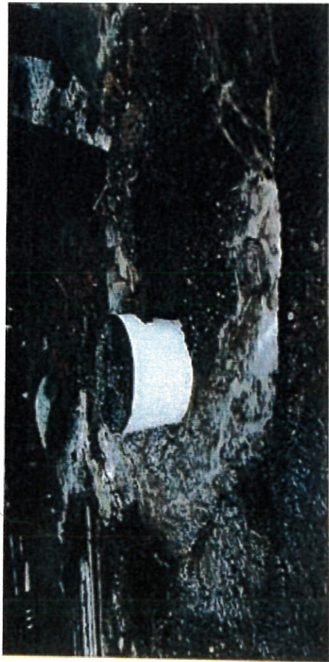
Photo 11. Eroded water utilities on West Reed Avenue.
