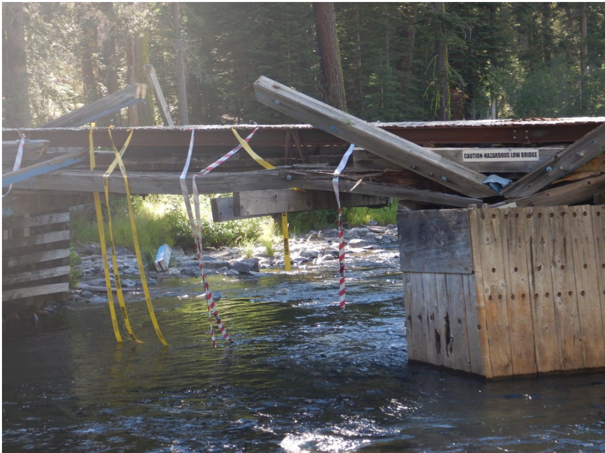
Figure 2.1—Photo of the collapsing bridge span with caution tape used to warn Truckee River recreators
