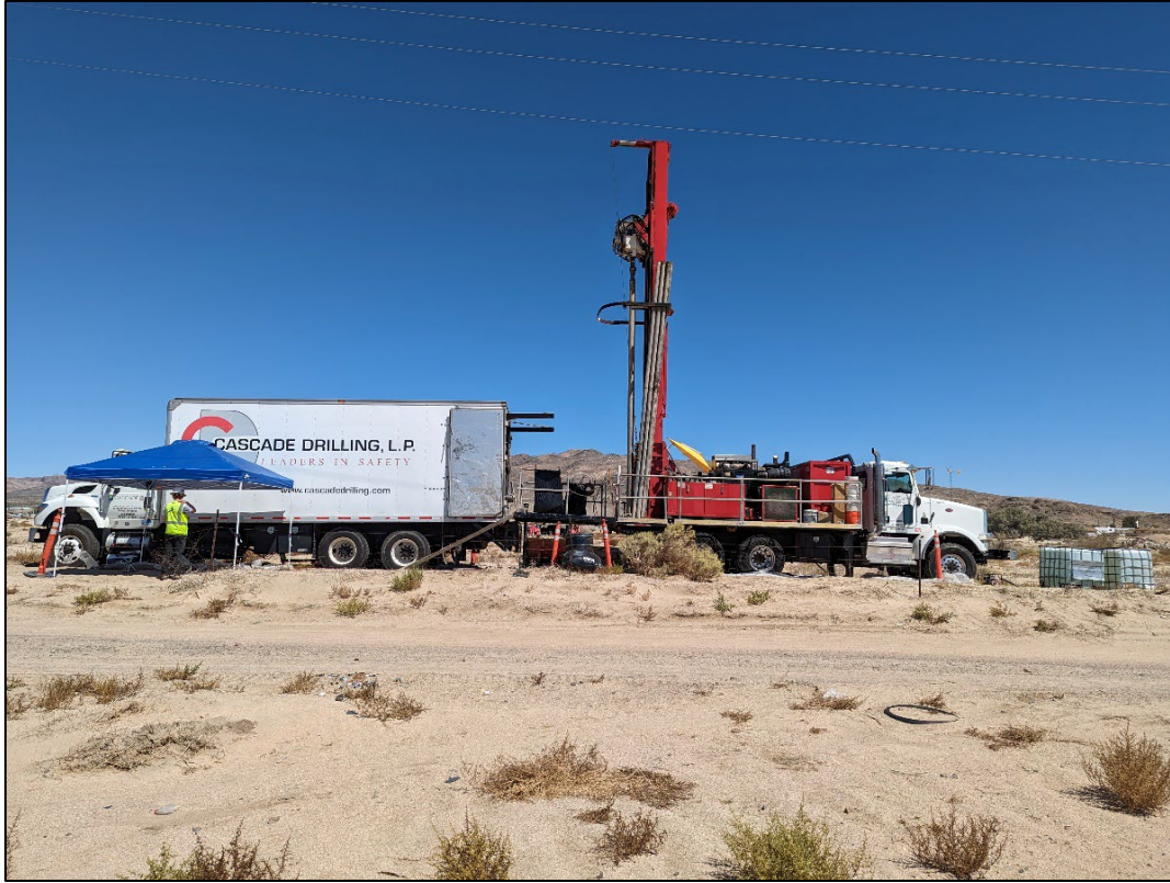
Figure 3.5: Drill rig from Cascade Drilling, L.P. during monitoring well installation on Crooks Avenue, August 2023
