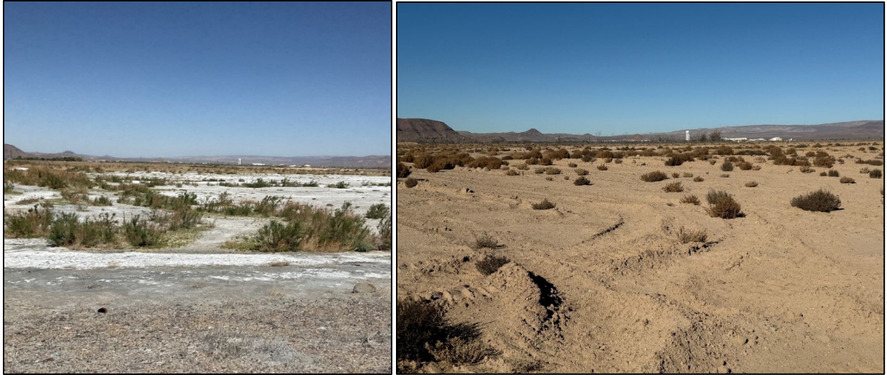
Photo 3.1: Before and after photographs taken from the southeastern side of the Facility looking northwest. On the left, salt and materials impacted from the Facility operations are visible. On the right, unimpacted materials are remaining after removal and consolidation.
