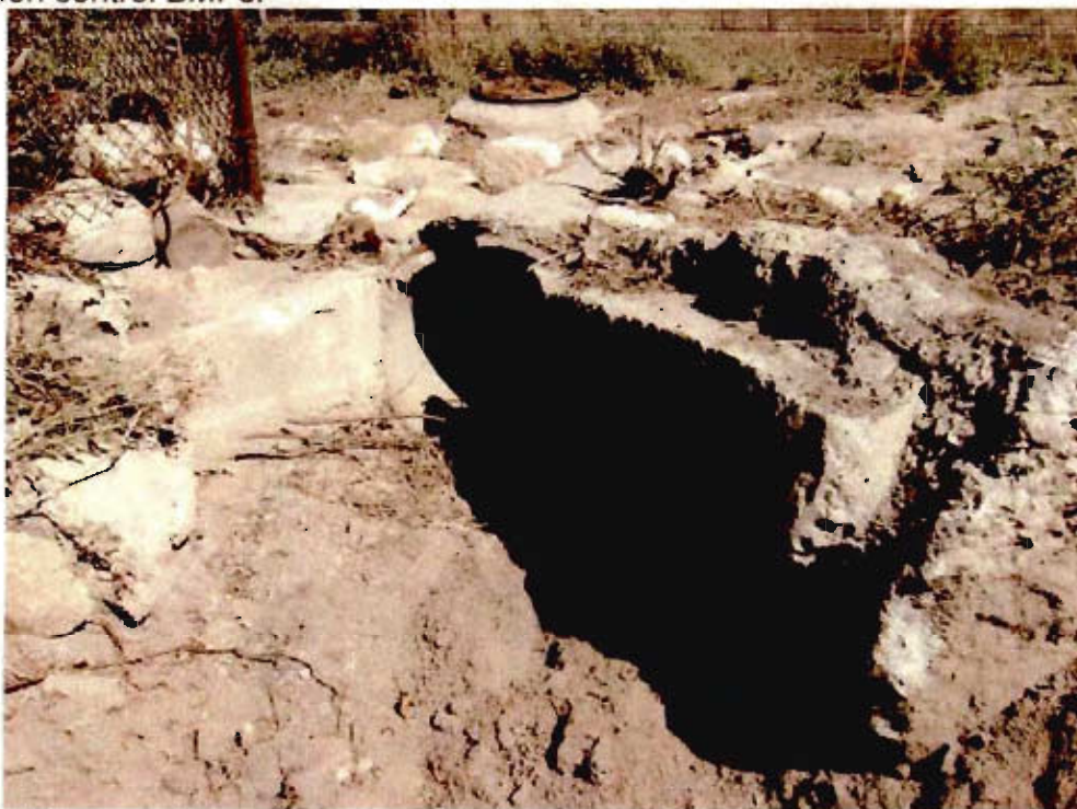
Photo 7. Onsite drainage enters an existing culvert in the northeastern corner of the site. This culvert discharges to a steep-walled canyon drainage.
