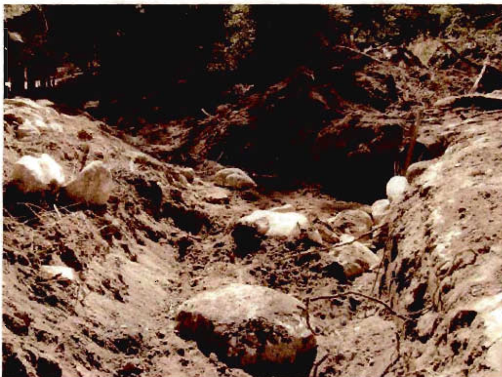
Photo 6. View upstream of natural drainage channel new culvert outlet to right of photograph. Note the grubbed vegetation and stockpiled soils and lack of stabilization or erosion control BMPs.
