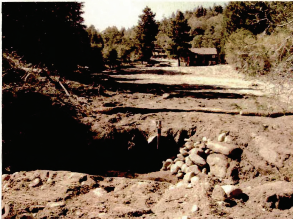
Photo 5. View looking west (upstream) across the site. The onsite culvert discharges to a natural drainage channel on the east side of the property (foreground). Rock cobbles and boulders placed on downstream side of discharge.
