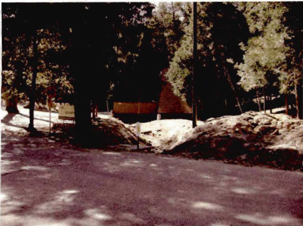
Photo 3. View of natural drainage channel upstream from site. Drainage enters culvert that discharges onsite (refer to photo 2).
