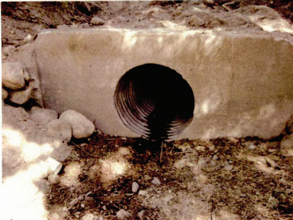
Photo 4. View of culvert and concrete headwall that conveys drainage across the site. This inlet is located approximately 10-feet downstream from the existing culvert discharge points in the southwestern corner of the site.
