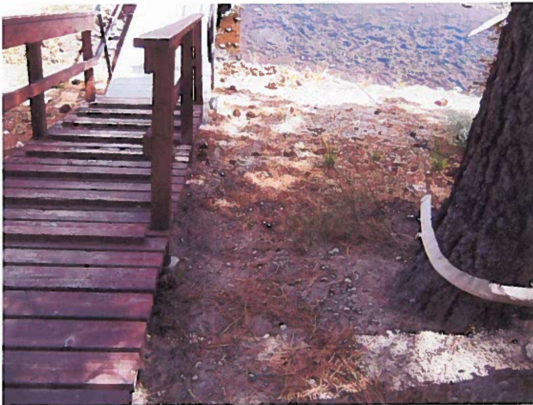
Photograph 24 – Close-up of the west side of the 4 th walkway shown in Photograph No. 20. Evidence of erosion can be observed.
