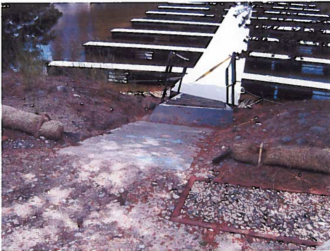
Photograph 10 – Moving closer to the ramp to get a further close-up of Photograph No. 08. Note that the fiber rolls do not prevent runoff from going down ramp and into marina
