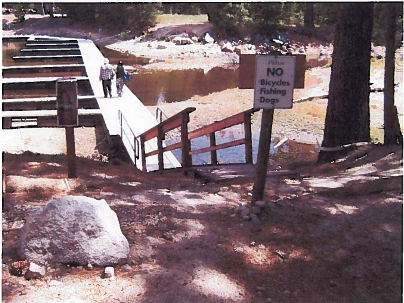
Photograph 20 - At 4th walkway ramp west of office. Fiber rolls to left of walkway and above walkway are not J-hooked at their ends. Fiber roll on right and above walkway is inundated with sediment, and evidence of sediment discharge into the marina is apparent.
