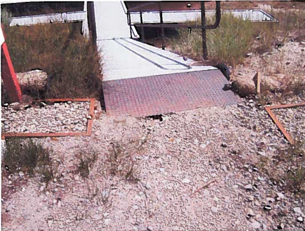
Photograph 17 - 3rd ramp west from office, facing south. A rill has formed beneath the metal plate, creating a threatened discharge of sediments into the marina. No fiber rolls or other BMP exists to prevent runoff from flowing down this area and causing bank erosion.
