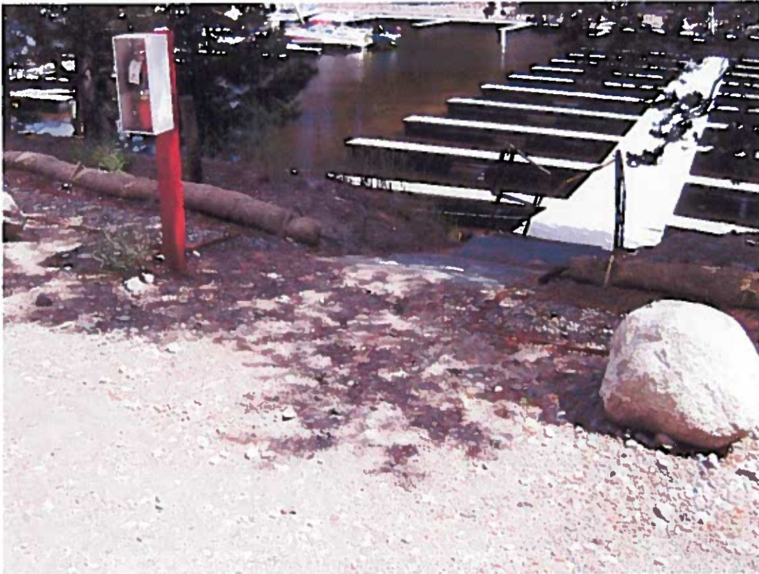
Photograph 09 – Close up of Photograph No. 08. Note that ends of fiber rolls are not J-Hooked.
