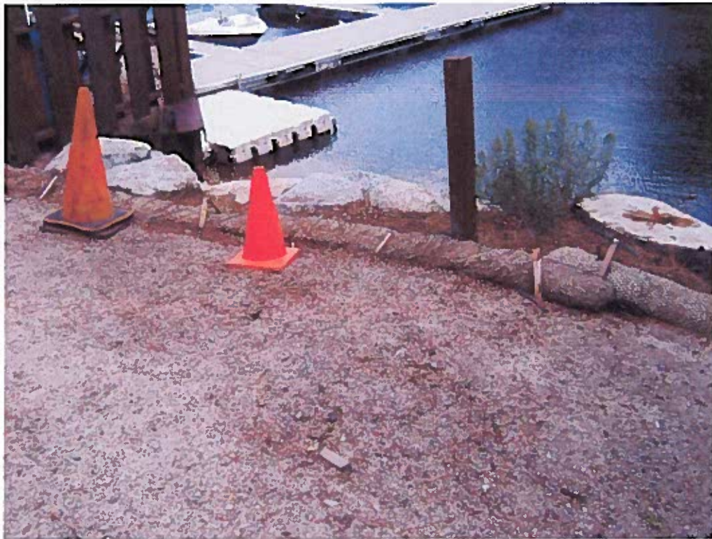
Photograph 06 - BMP joint is not J-hooked, and the fiber roll section by the pilings has been flattened. This area is by marina office, facing southeast
