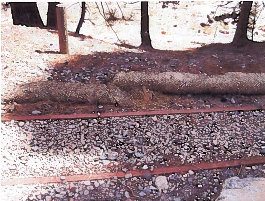
Photograph 18 - Midway between 3rd and 4th ramps west of office. The ends of the fiber rolls are degrading, and they are barely overlapped.
