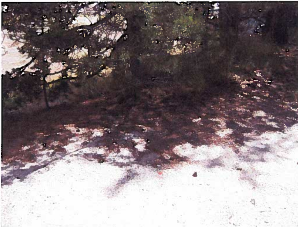
Photograph 30 - Standing at photo point 28, panning west from photo point 29, looking southwest-west. Fiber rolls have not been placed to collect potential stormwater runoff from the unpaved parking area.
