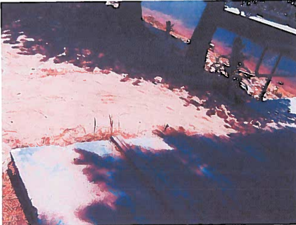
Picture 4: This is gangway number 1, closest to the lake. Due to the topography of the parking lot, a low spot forms at the top and runs down during significant rain events.
