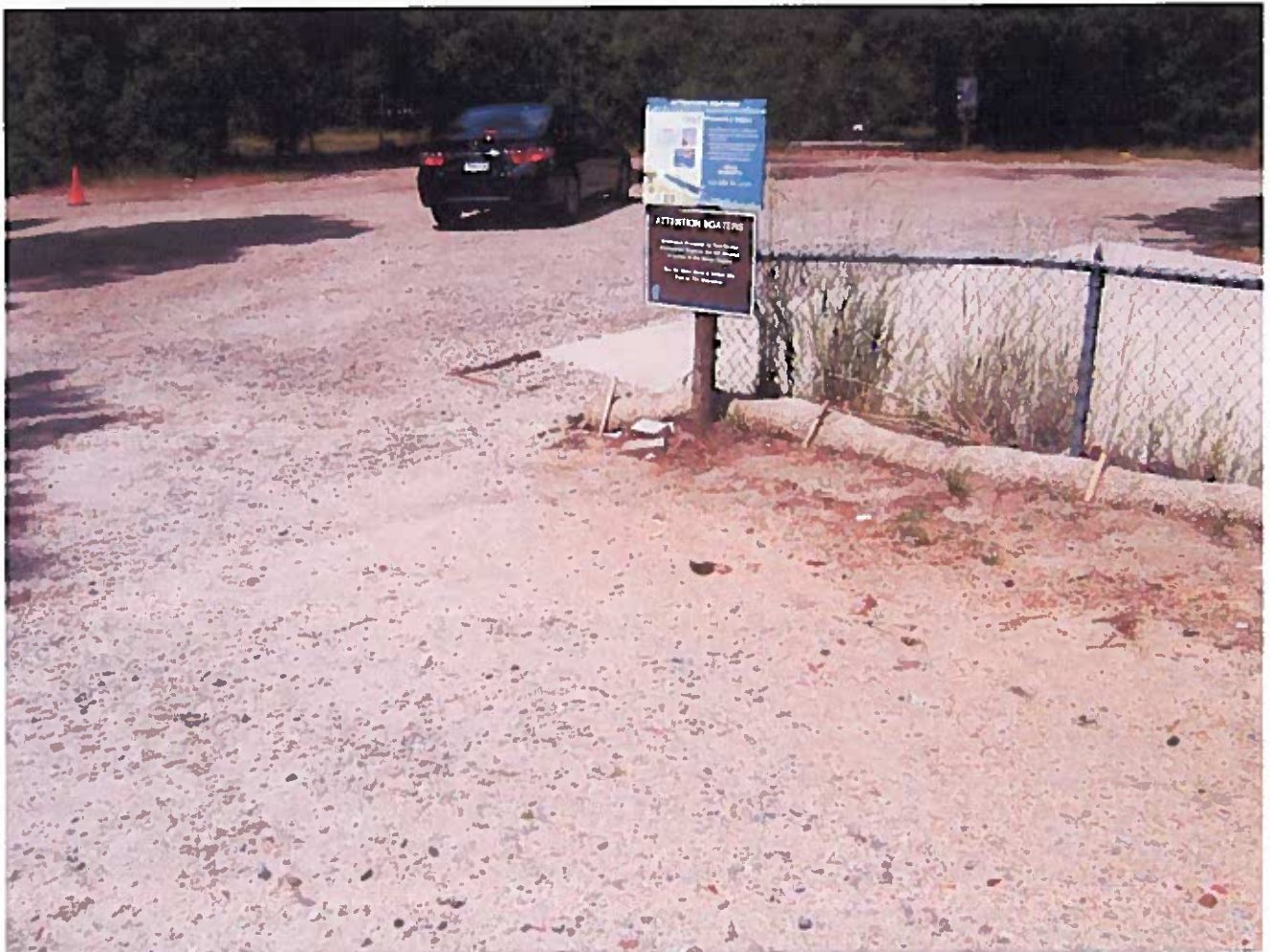
Photograph 04 - Looking East, Northeast at fiber roll. The fiber roll is not J-Hooked at its end which is also installed perpendicular to the grade lower than the rest of the fiber roll, and not parallel to the grade. Any runoff that flows toward the fiber will flow along it toward the downgradient end and, eventually, down the boat ramp and into the marina.
