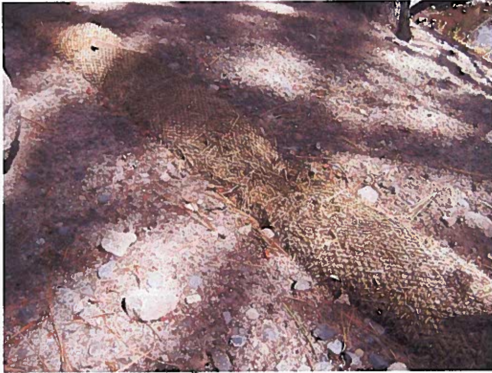
Photograph 25 - 10 feet west of the 4 th walkway west of the office. The fiber roll has degraded.
