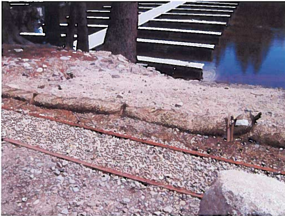
Photograph 15 - About 20 feet west of 2nd ramp west from office, looking south-southeast. The fiber roll has been degraded degraded and flattened.
