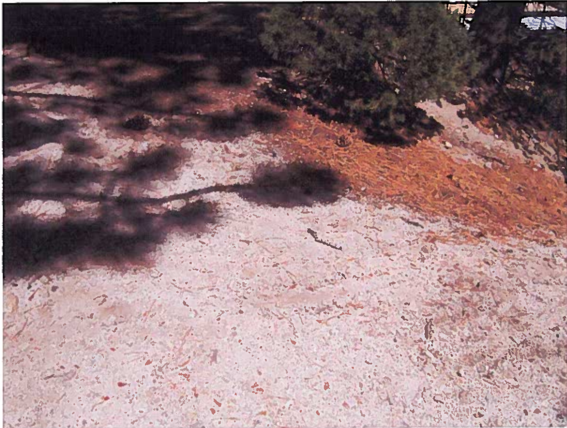
Photograph 26 - 20 feet west of 4th walkway ramp from office, facing east. No fiber roll has been installed, and a small gully erosion can be observed.
