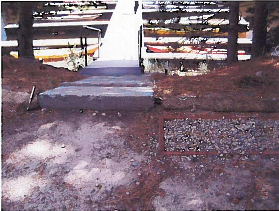
Photograph 07 - First ramp west of office, facing south. A gap exists between the concrete section of the ramp walkway and the fiber roll to the right (west) of the ramp. Runoff that bypasses the drainage ditch will flow through this area and into the marina.
