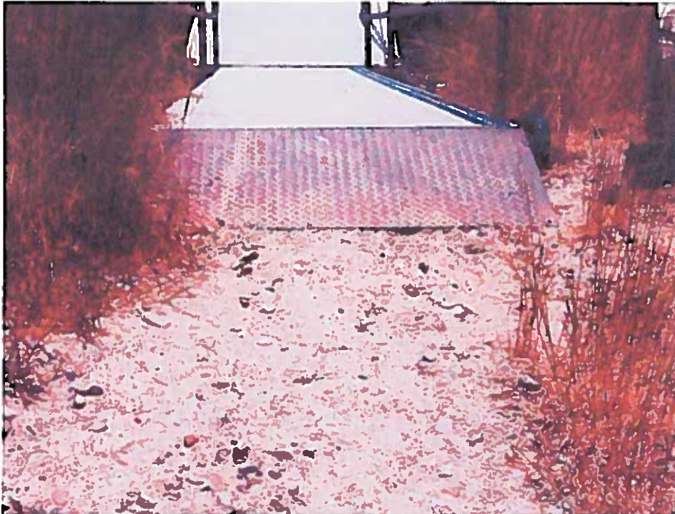
Picture 2: The walkway is downward sloping from the parking lot to the gangways. Potential for rill or gully erosion into the marina surface waters is possible.
