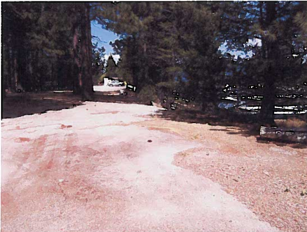
Photograph 32 - At west end of the marina boundary in the boat trailer parking area looking east. Fiber rolls were not installed at trailer parking area. Note the evidence of ponded water in the middle of the photograph, indicating fiber rolls may not be necessary in this area.
