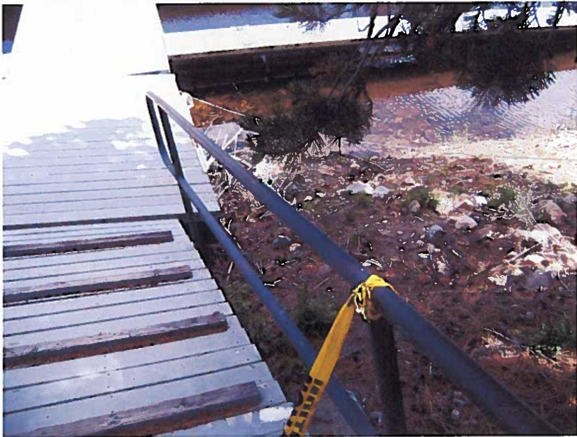
Photo 14 – From same location as Photograph No. 13, but looking on the west side of the second ramp west of office.
