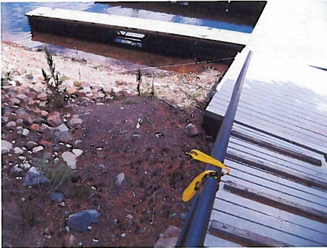
Photograph 13 – Close up of sediment deposit noted in Photograph No. 12.
