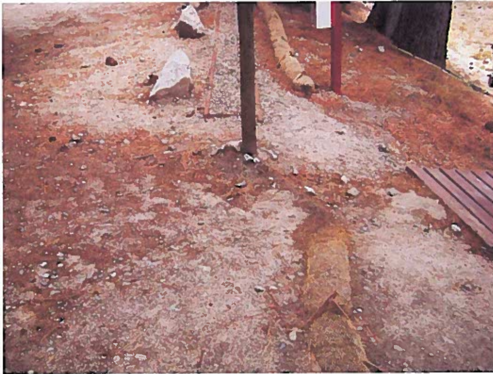
Photograph 23 - Close up of the sediment-inundated fiber roll shown in Photograph No. 20, facing east. The fiber roll end in the foreground was slightly J-Hooked to capture runoff and sediment, while the end of the fiber roll at the top of the photograph is not J-Hooked and allows runoff to flow down the embankment. Photograph taken by Will Chen.
