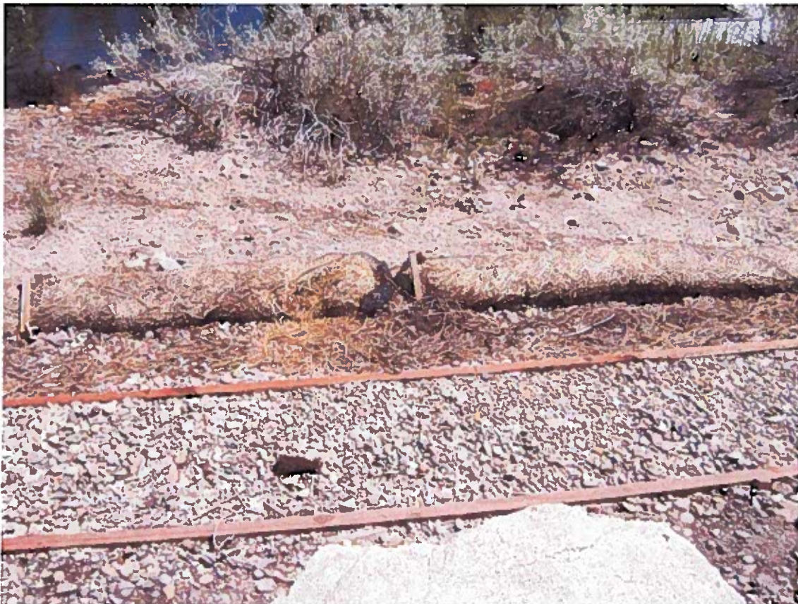
Photograph 16 - Mid-way between 2nd and 3rd ramps west from the office. The fiber rolls have been slightly flattened, and the ends have not been overlapped leaving a gap between the rolls where stormwater runoff can become concentrated.
