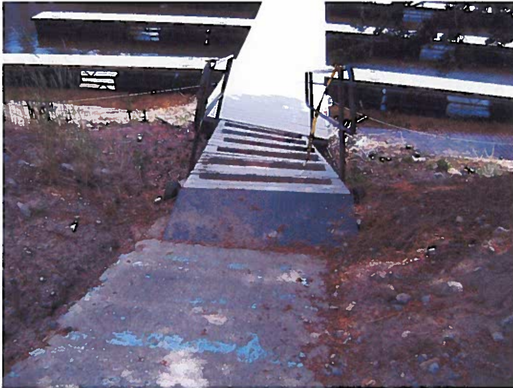
Photograph 11 – Moving closer to the second ramp west of office to get a further close up.
