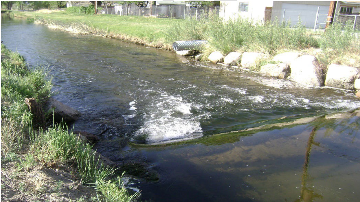
Photo 7-1 Concrete encased clay pipe submerged in water at a canal crossing. City of Bishop planned to replace this 15-inch clay pipe with a new 18-inch plastic pipe (more
