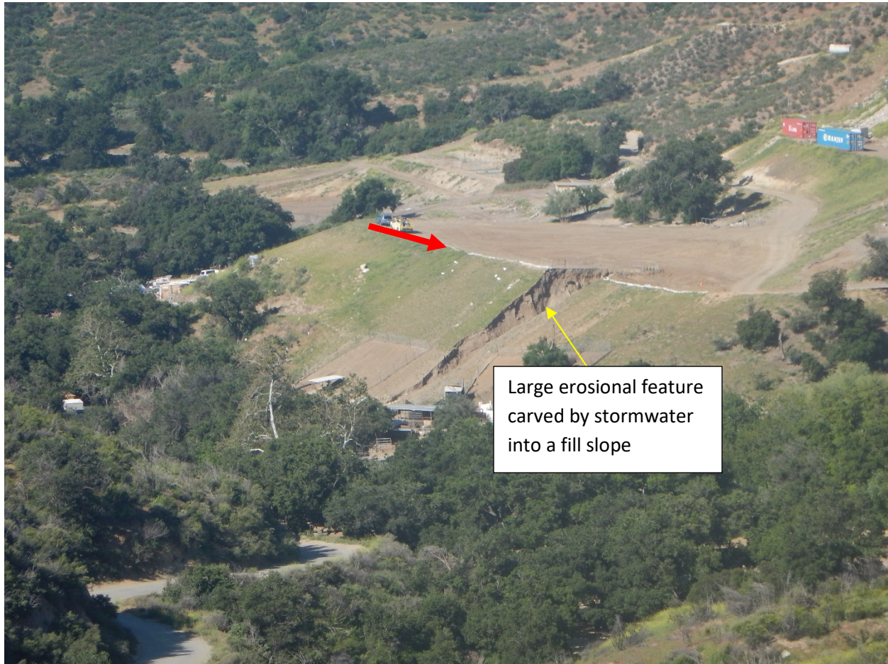
Photo 3. View looking southwest from Photo Location 1. Showing canyon carved into slope in parcels 2821-009-030 and 2821-009-031, which are owned by Mr. Wayne Fishback and Cepheid V, LLC respectively. The base elevation of the large erosional scour is in the immediate vicinity of the Ybarra Creek bed. It can be inferred from this photo that all the stormwater scoured fill materials were transported into Ybarra Creek. The red arrow indicates the remnant sandbag wall, presumably the wall that Mr. Fishback alleges was sabotaged. The photo was taken at Longitude -118 36 21.75 and Latitude 34 18 22.79 on April 12, 2017.
