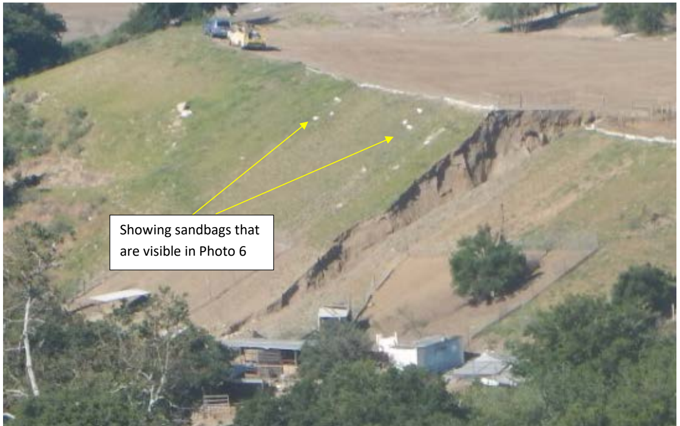
Photo 4. View looking southwest from Photo Location 1. Close up of Photo 3. Showing the sandbags from the sandbag wall that have fallen down the fill slope. These sandbags are visible in Photo 6 and were present during the October 17, 2016 Inspection.
