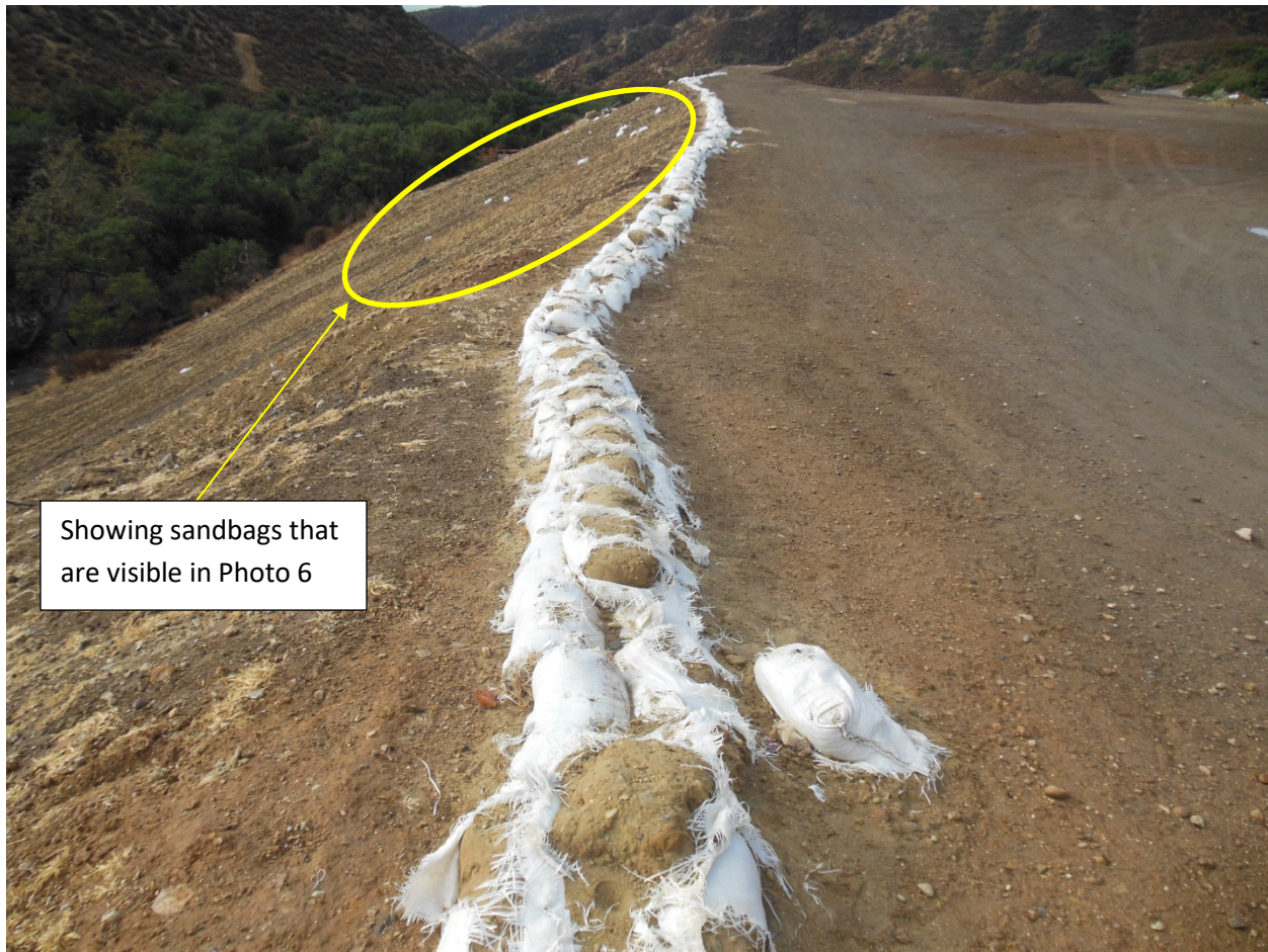
Photo 6. Close up of the sandbag wall along the slope break of the fill slope in Photos 3 and 4 during the October 17, 2016 inspection. The sandbag wall is above the large erosional scour that later developed during the February 2017 rainstorms. The photo shows that number sandbags from the sandbag wall have already fallen down the fill slope. The photo also shows that the sandbags, as of October 17, 2016, were deteriorated and releasing sediment so that they could not function as an effective best management practice (BMP) for subsequent winter storms.
