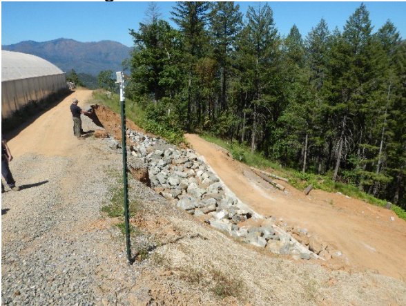
Photo 27: View of lower landslide P10 and rocking to minimize additional failure.
