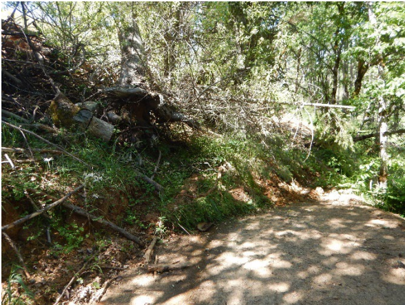
Photo 21: View of landslide movement on road below P8.
