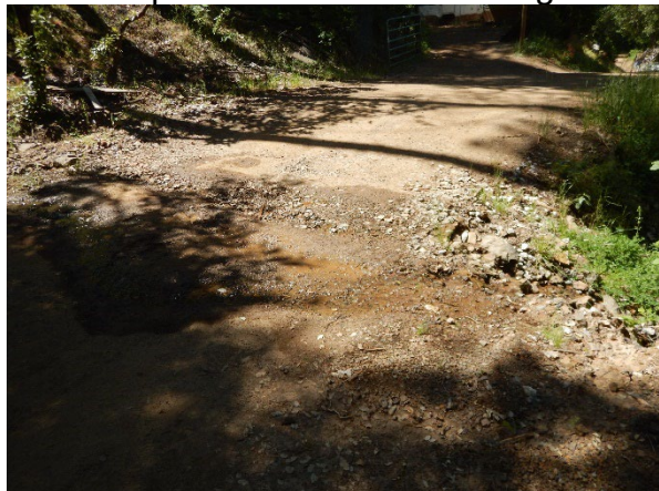
Photo 6: Water flowing across road at undeveloped watercourse crossing P2.
