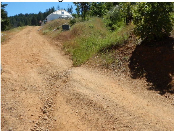
Photo 23: View of flow path across road at P9 west of greenhouses.
