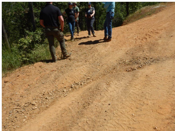
Photo 24: Continued view of P9 flow path across the road.
