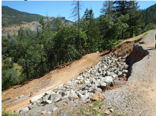
Photo 28: View of lower landslide P10 looking East.
