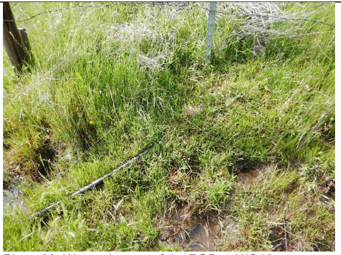
Photo 28: Water pipe out of the POD at WQ18
