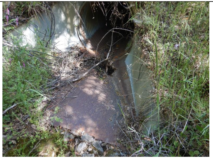
Photo 22: Inlet of a partially rusted culverted watercourse crossing at WQ14
