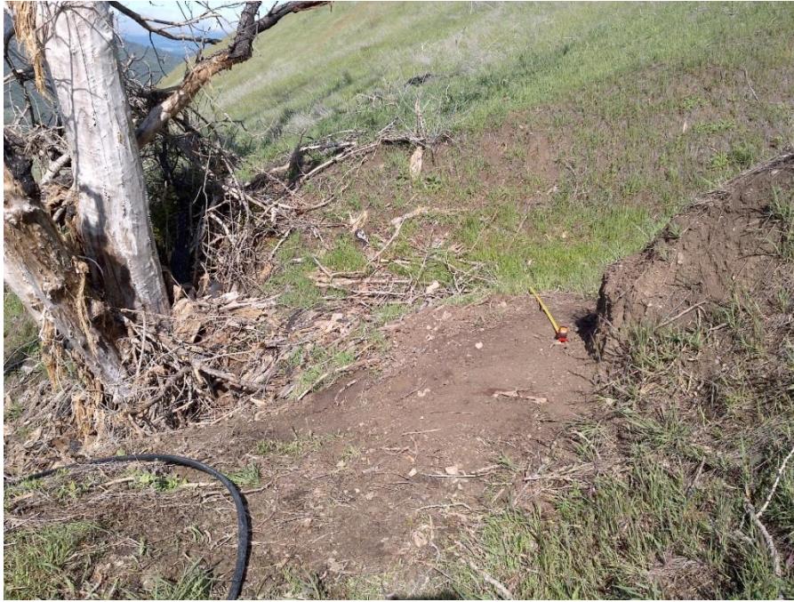
Figure 12—Looking west where an earthen pad extends into the watercourse at WQ5. The dead tree in the left of the image is also visible in the previous image. Approximately 18 cubic feet of earthen fill has been placed into the channel; a patch six feet square averaging six inches deep.
