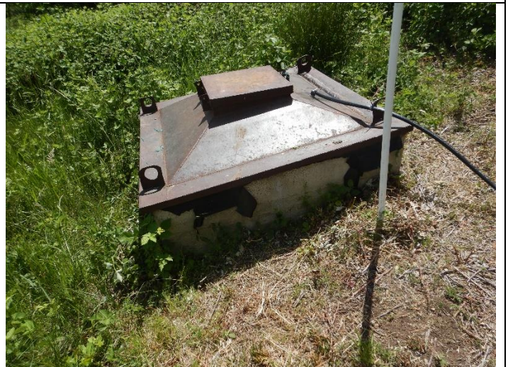
Photo 12: A second water storage structure connected to a water supply pipe in the vicinity of WQ9
