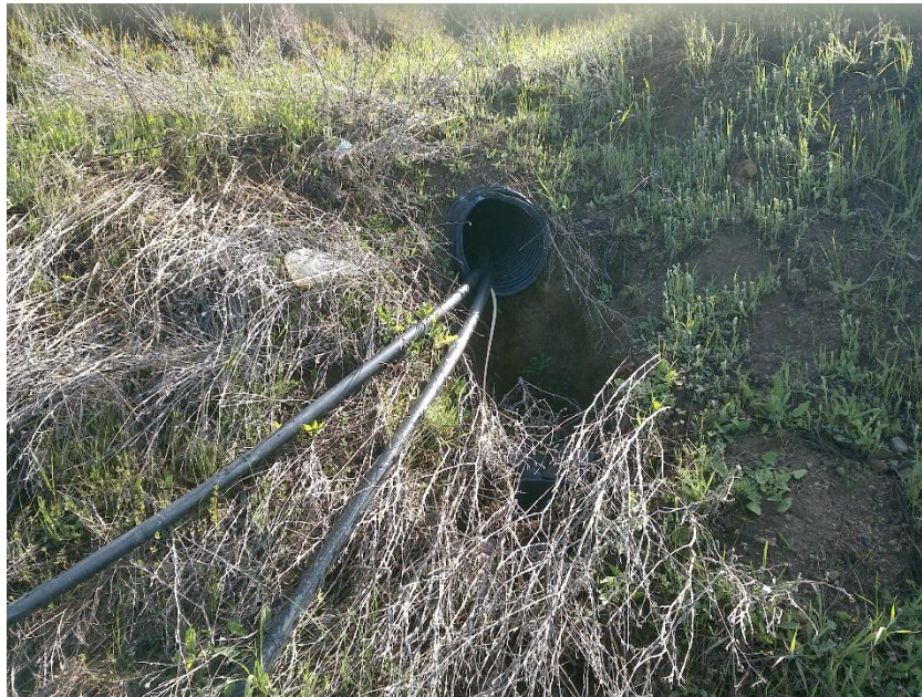
Figure 10—Looking north at culverted watercourse crossing at WQ4. The culvert is perched approximately two feet above the channel bed.
