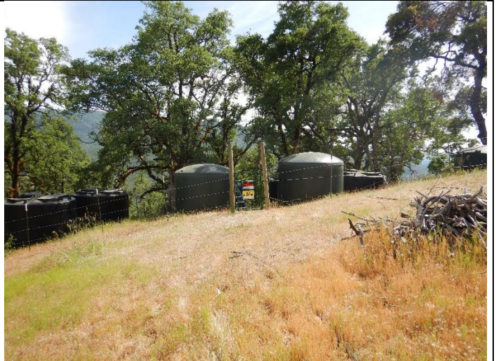
Photo 26: Water storage tanks at WQ17
