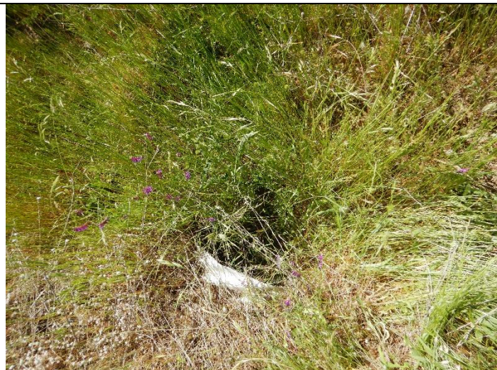
Photo 24: Inlet of a culverted watercourse crossing at WQ15, appears to be functioning well but needs clearing of the vegetation
