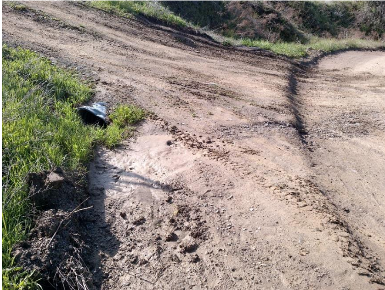
Figure 4—Looking south at WQ1 at the intersection of the gated access to the Property to the left and the shared-use access road to the right. The road has been graded such that stormwater will flow across the road instead of through the culvert pictured in the left of the image.
