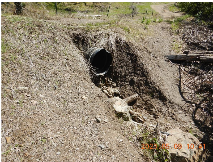
Figure 25—Reservoir outlet drain at WQ9 directed toward USGS mapped blueline stream out of view to the right of the image. The outlet pipe is 20-inches in diameter and lacks armor which has resulted in erosion and downstream transport of the earthen fill.
