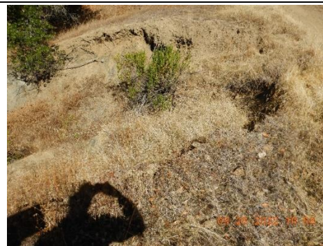
Photo 32 – collapsed roadside fill prism at inspection point WQ20
