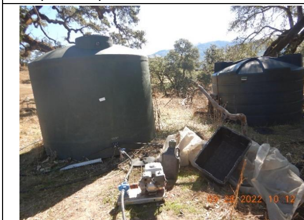
Photo 25 – water storage tanks, improperly stored gasoline tank and pump at inspection point WQ10
