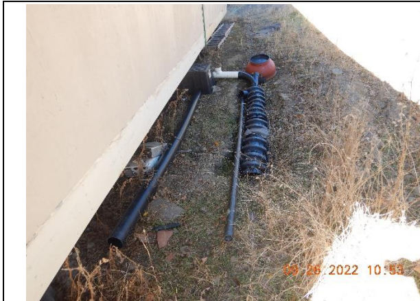
Photo 33 – Domestic wastewater pipe near a class III watercourse at inspection point WQ19
