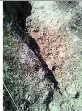
Photo 8 - Pond embankment erosion threatening sediment delivery at inspection point WQ30
