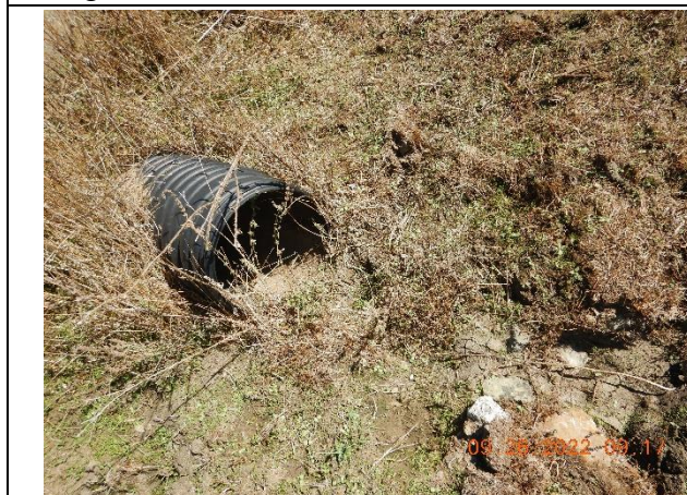
Photo 9 - Culvert outlet delivering sediment to surface water at inspection
