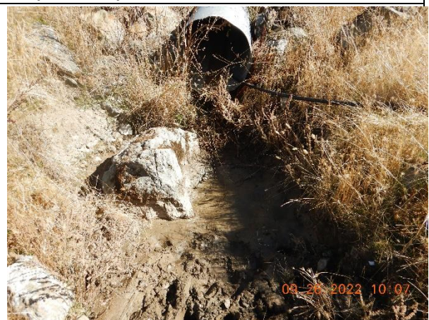
Photo 10 - Culvert outlet showing sediment delivery at the stream
