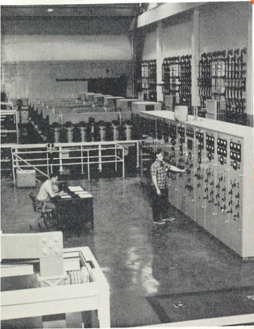
Mercury arc rectifiers, which are typical of the extensive electrical installation necessary for a continuous supply of energy.
