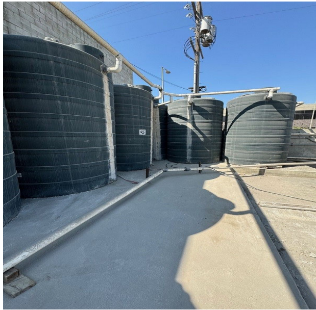
7 Figure 4. Sun Valley Storm Water Runoff Capture System
