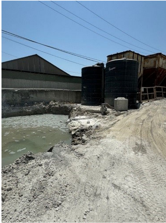
Figure 7. Downey Storm Water Runoff Capture System
