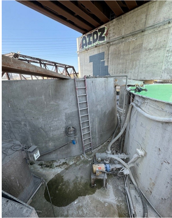
1 Figure 3. Los Angeles Facility Storm Water Runoff Capture System
