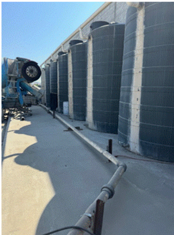
Figure 6. Sun Valley Storm Water Runoff Capture System
