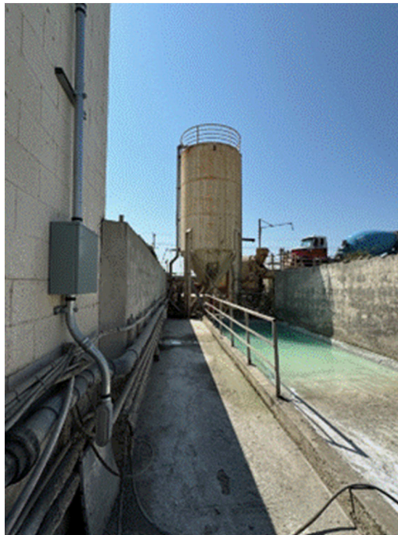
Figure 5. Sun Valley Storm Water Runoff Capture System
