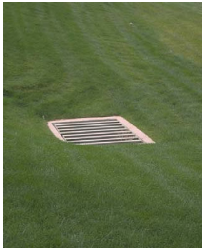
Photograph ST-6—Field inlets frequently need maintenance.
