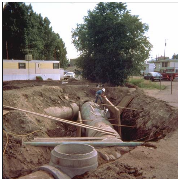
Photograph ST-2—The capital costs of storm sewer construction are large, emphasizing the importance of sound design.
