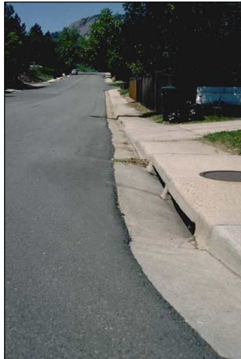
Photograph ST-1—The critical role that streets play in urban inlet and storm sewer drainage is often not properly taken into account.
