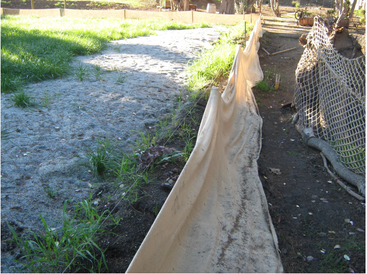
Sagging Fence and Saturated Soils 12-16-15
