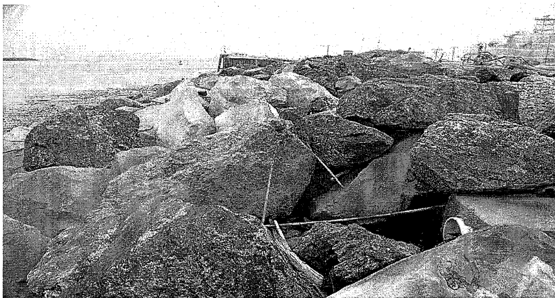
Figure5: SDTF facility outfall consisting of 12-inch conduit positioned on rock rip rap at a distance of thirteen feet from receiving water.
