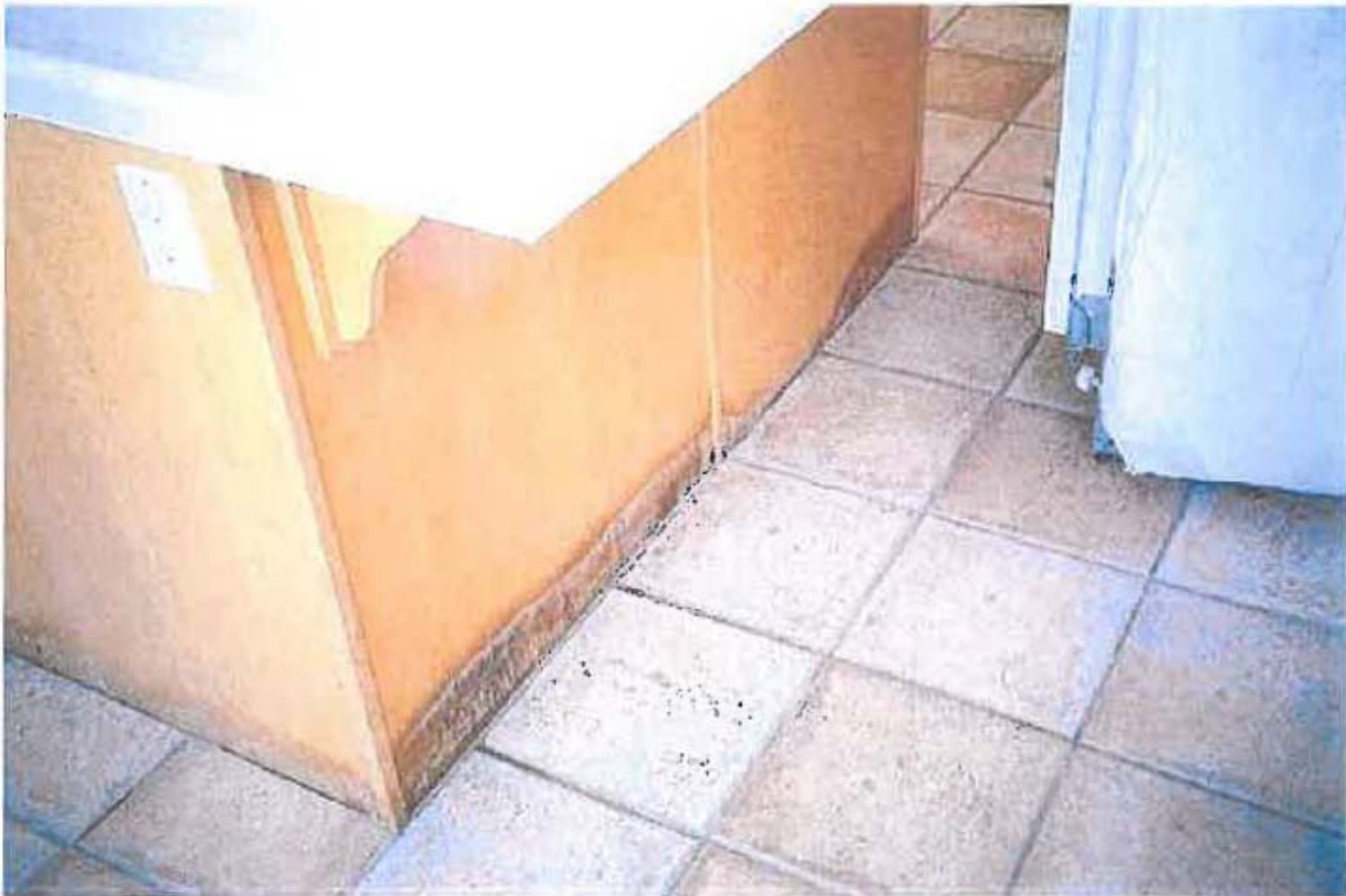
Photo 4- water migration through slab into cabinetry
