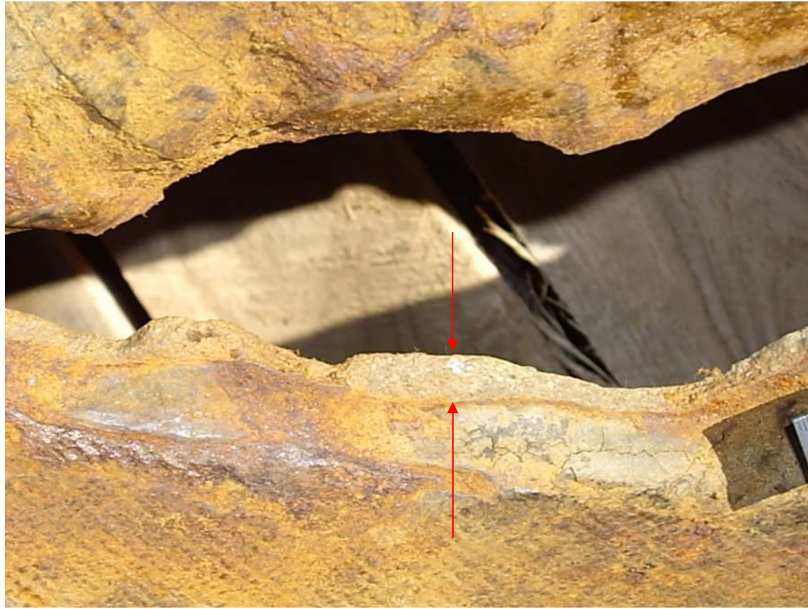
Figure 4 - Corrosion hole close-up
