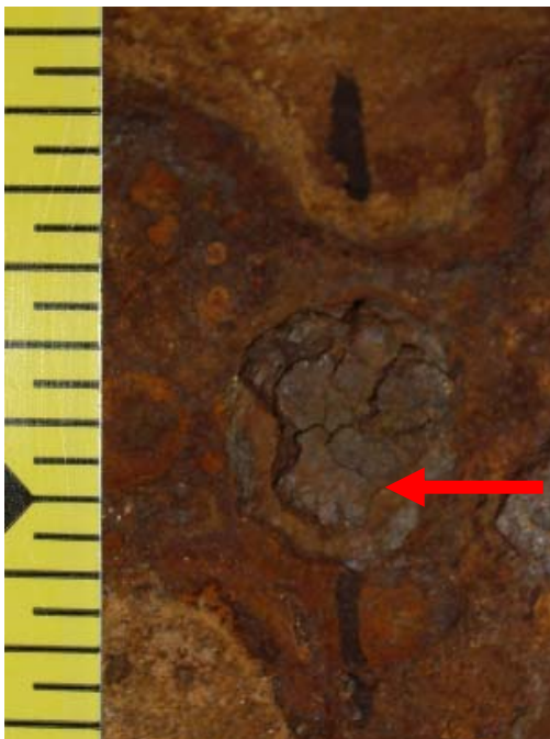
Figure 8 – Close up of corrosion product
