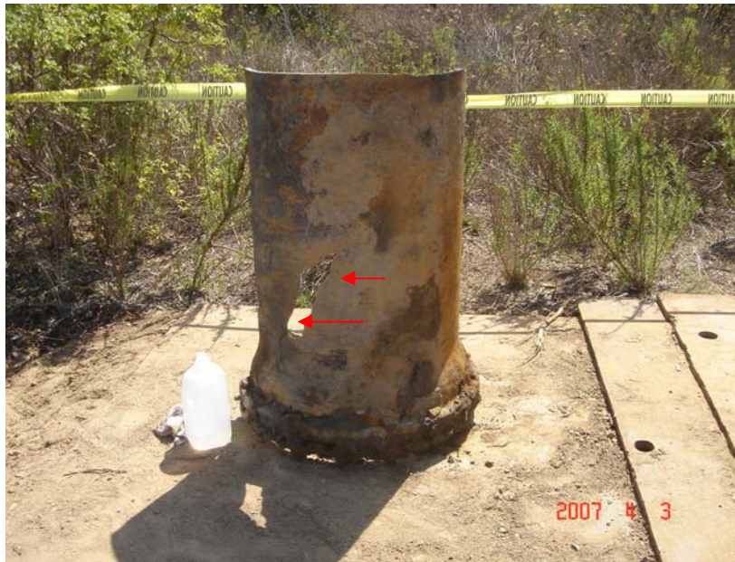
Figure 2 – Sectioned pipe with failure (below springline)
