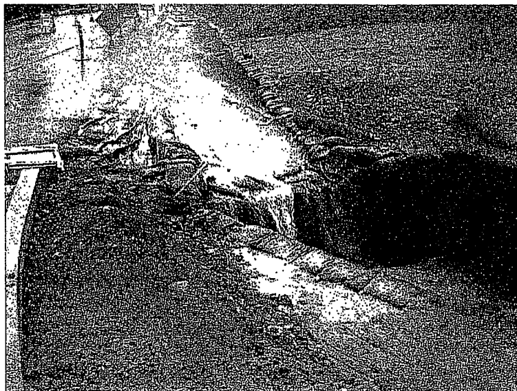
152. This is the culvert entrance to photo 151 on the south side of Avenue of Nations receiving sediment-laden runoff.
