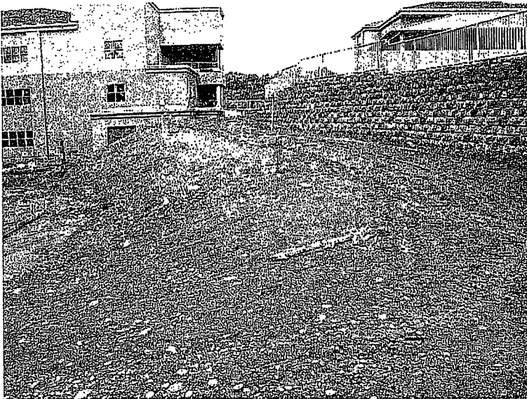
192. A slope has no erosion or sediment controls. A construction access road has no sediment controls.
