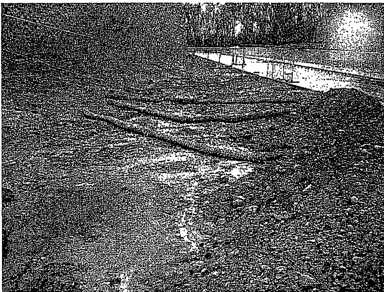
154. Upstream of the culvert entrance on the western side, no erosion controls have been implemented. Fiber rolls have not been trenched in and staked therefore they are doing little to stop the sediment flows.
