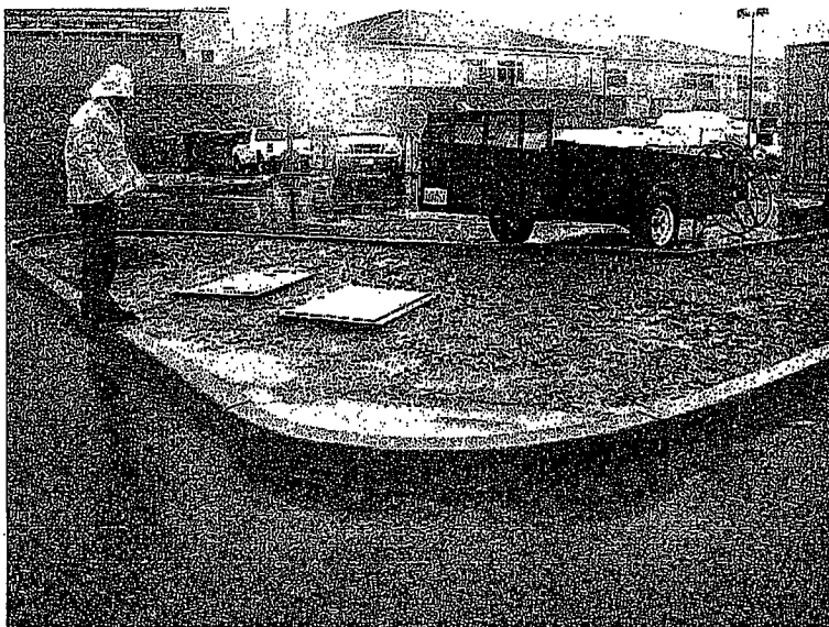
164. Medians in the school parking lot did not have any sediment controls.
