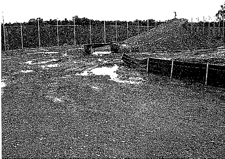
174. Silt fence around a stockpile is damaged and missing.
