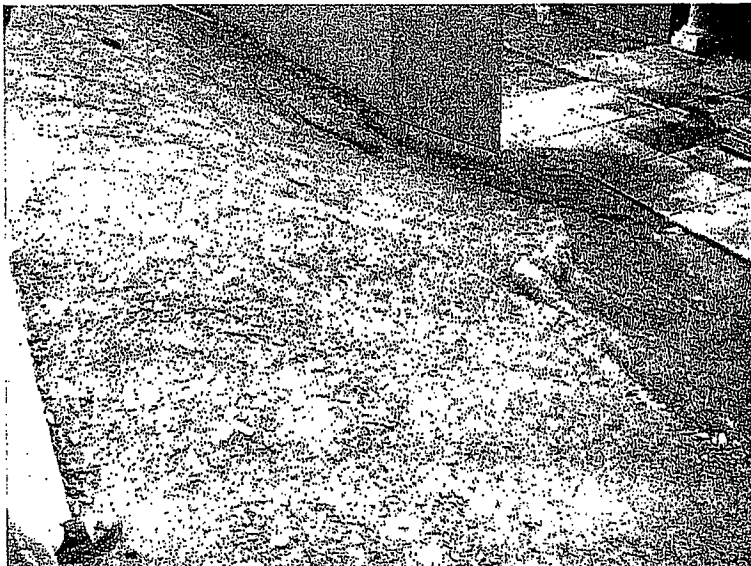
188. A slope with inadequate sediment controls. The fiber roll has failed. An erosion gully is running along the slope next to the wall.
