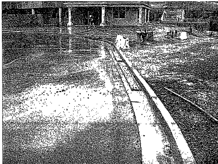
166. Sediment is tracked onto the street. No sediment controls have been implemented behind the curb.
