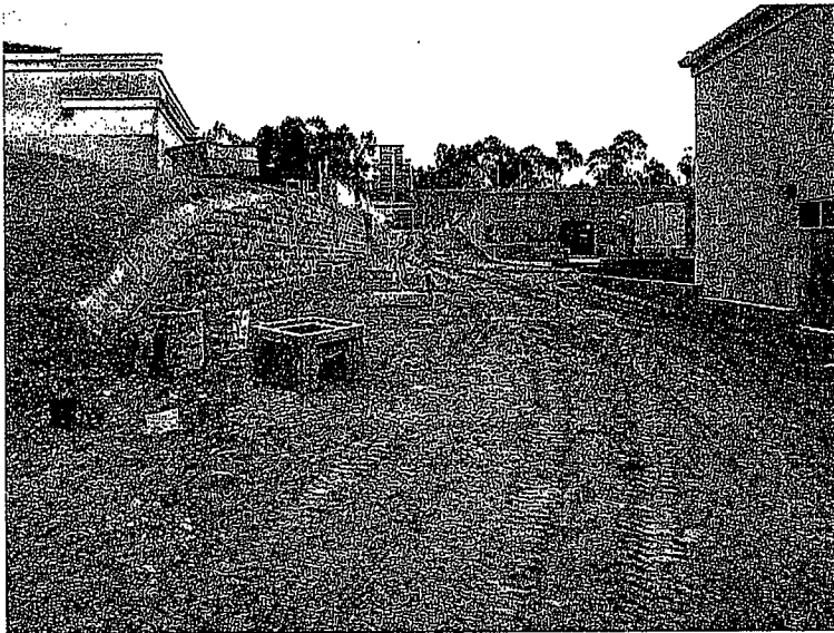
201. A construction access road with no sediment controls.
