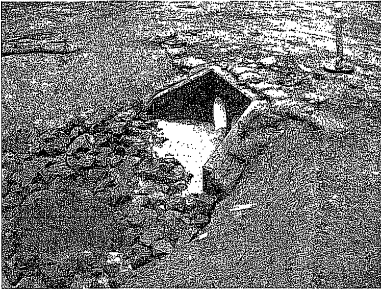
151. A closer look at the storm drain culvert discharging the sediment-laden runoff.
