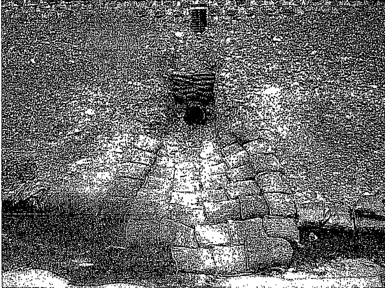
156. A runoff discharge point upstream to the east of the culvert in photo 153. Sediment-laden runoff flows out of the pipe across the gravel bags and into the plastic lined ditch.
