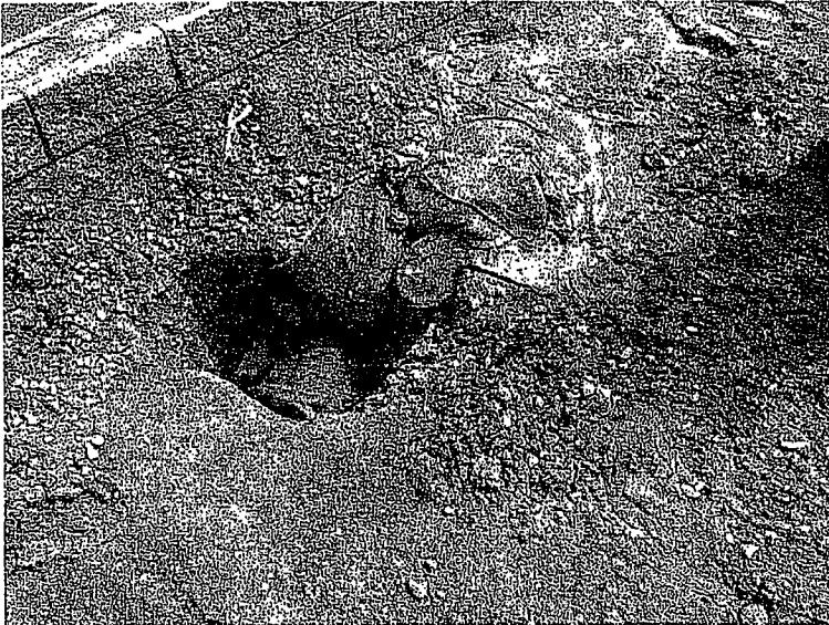
187. Storm drain inlet that is covered with filter fabric and gravel bags has been overwhelmed by sediment flows.
