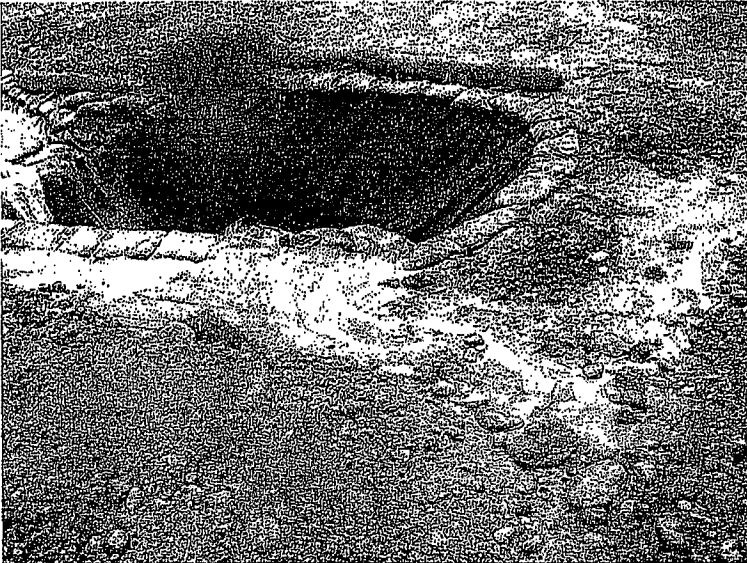
153. Another view of the culvert entrance on the south side of Avenue of Nations, shows sediment and sediment-laden water entering the storm drain culvert from another side.
