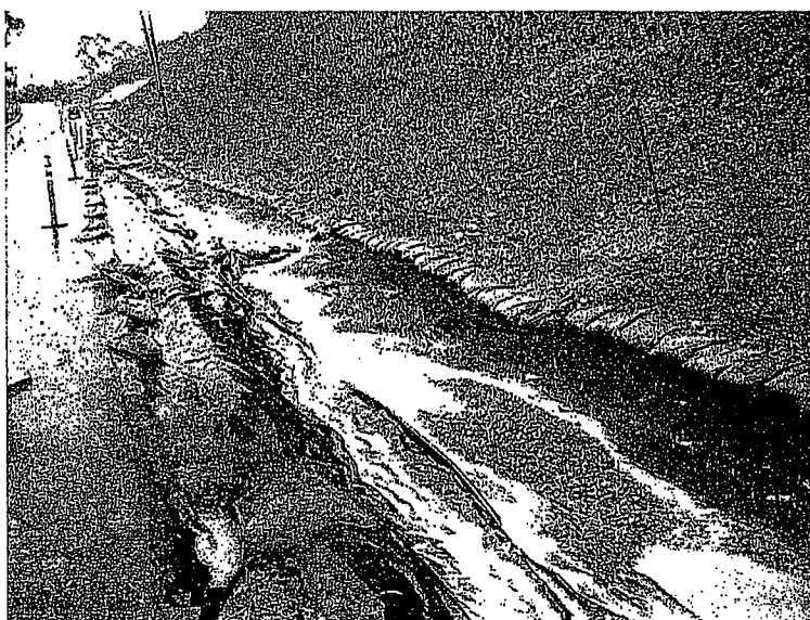
157. This plastic lined ditch is along the south side of the Avenue of Nations. The ditch terminates at the culvert in photo 153. Inadequate sediment controls along the face of the slope and the toe of the slope. Sediment laden water and sediment in the ditch.
