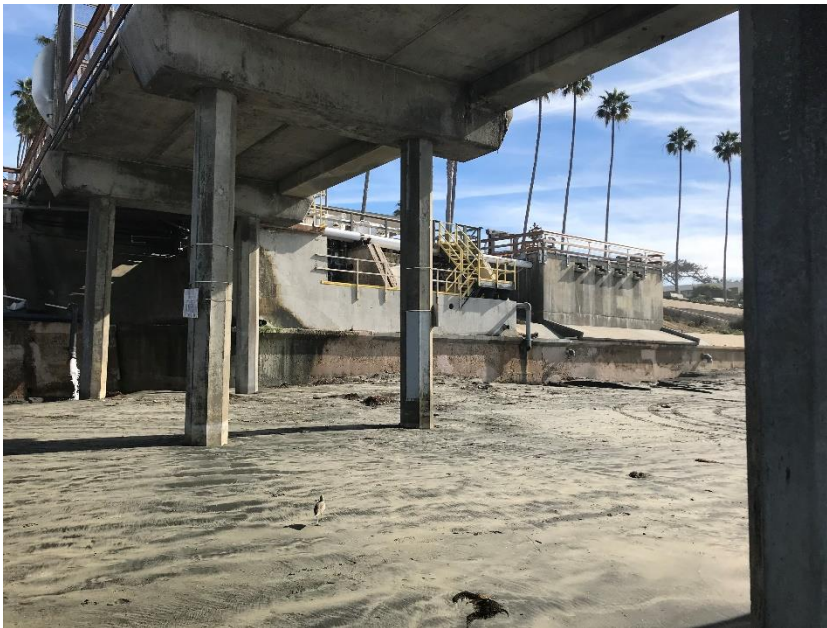
Photo 6: Photo provided by Kimberly O' Connell of University of California San Diego on January 30, 2020, showing bottom of the pier. Note that there is no sand displacement or loss below the pier.
