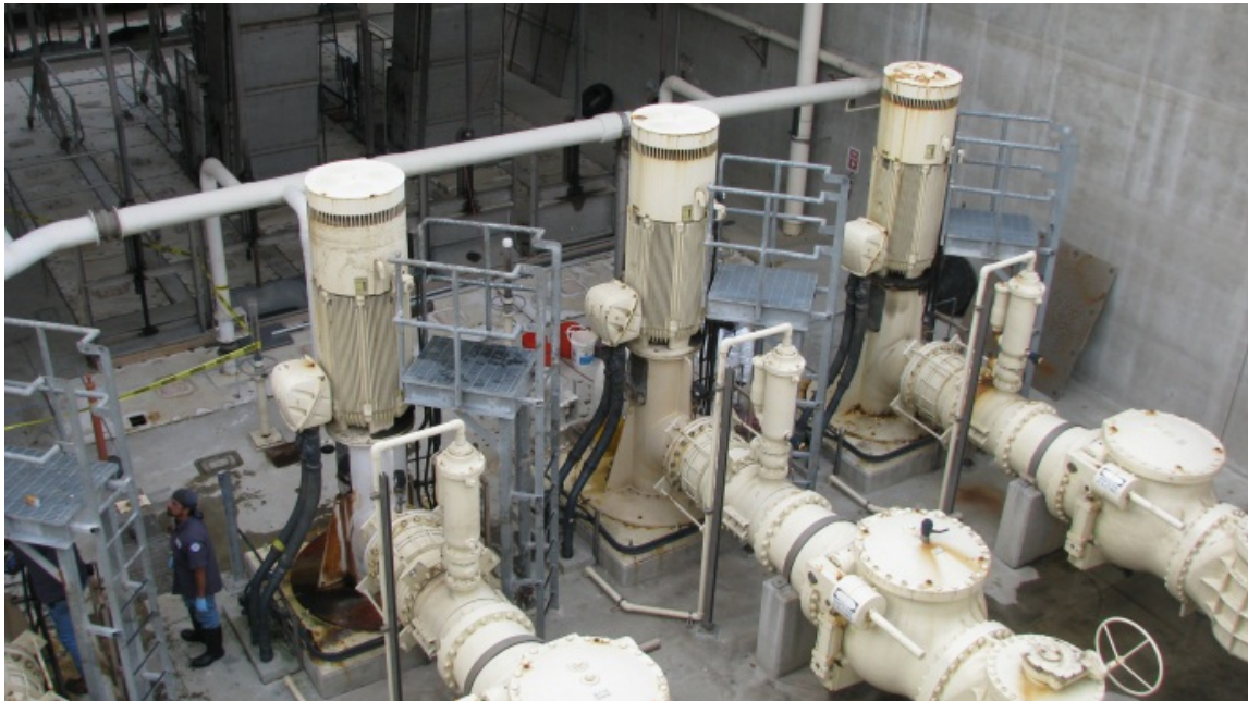
Figure 2: Pump motors showing high water mark at vents on top of motors. April 5, 2012
