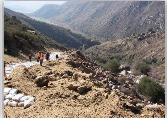
Photo by: State Water Board staff.
