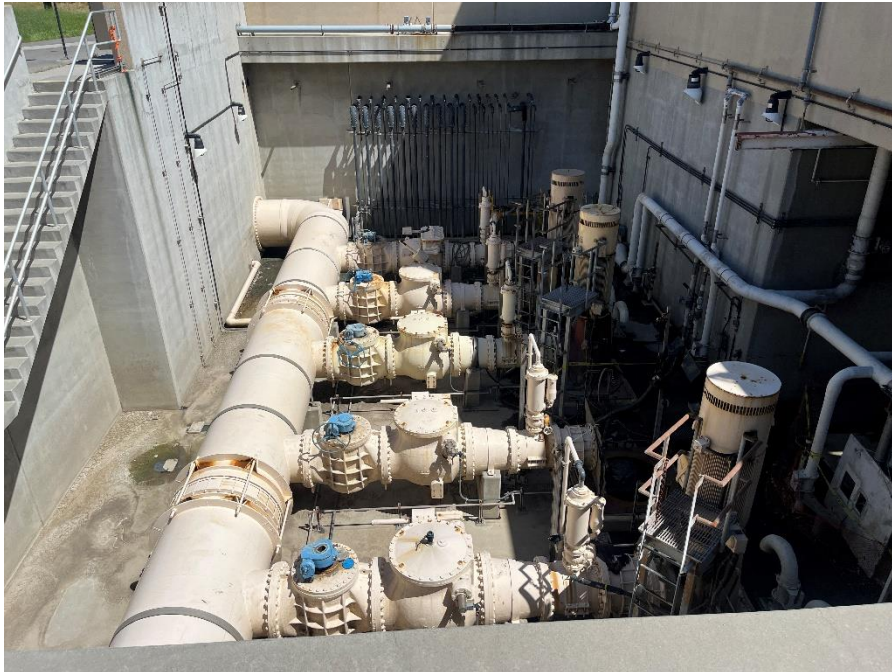
Figure 3: Influent pumps. (MC 04/03/2024)
