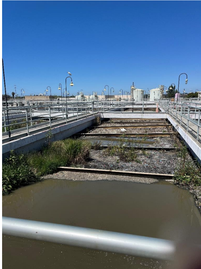
Figure 8: One of four inoperable PSTs. (MC 04/02/2024)
