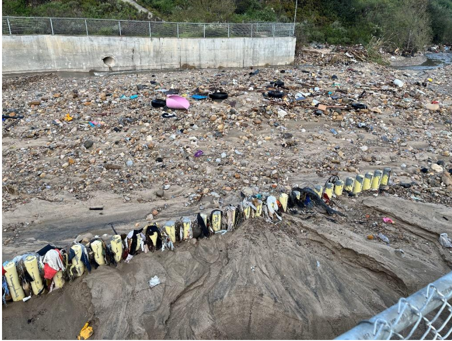
Figure 1: Trash and sediment at Smuggler's Gulch Canyon Collector. Bollards are approximately five feet in height. (Veolia 04/01/2024)
