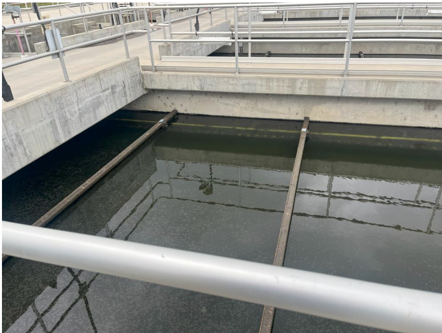
Figure 10: Secondary settling tank. (MC 01/10/2024)
