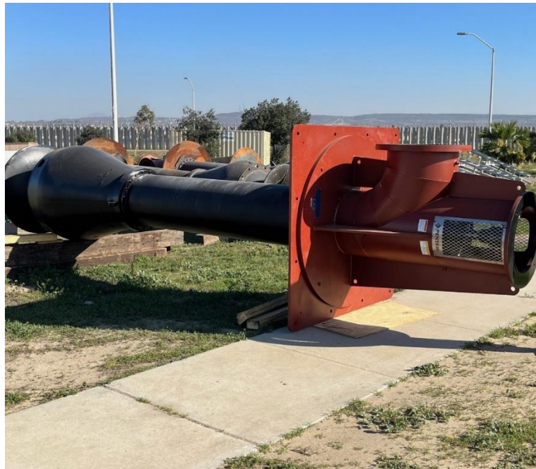
Figure 5: Closer view of one of the new influent pumps. (USIBWC 12/13/2023)
