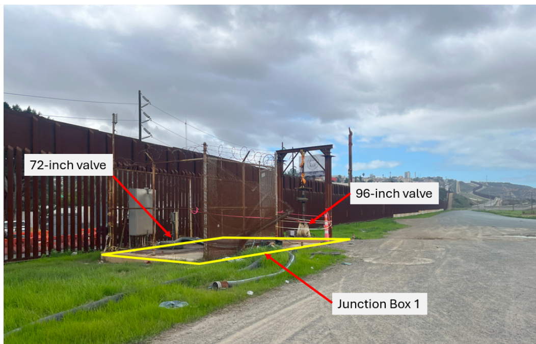
Figure 2: Junction Box 1. (MC 01/10/2024)
