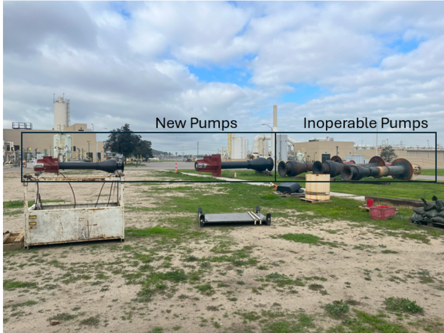
Figure 4: Two new influent pumps on the left. Three inoperable influent pumps on the right that have been removed for replacement. (MC 01/10/2024)
