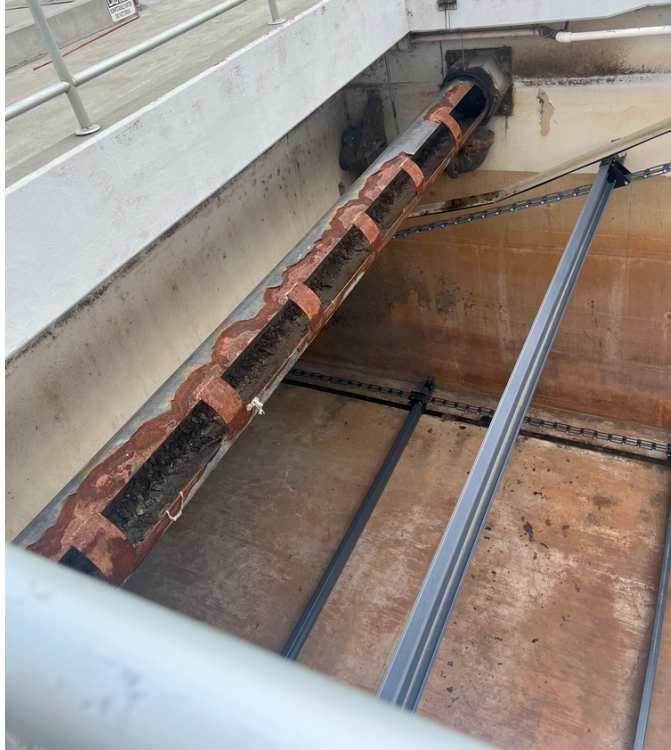
Figure 7: Skimmer trough at PST No. 5. prior to resuming service (MC 01/10/2024)
