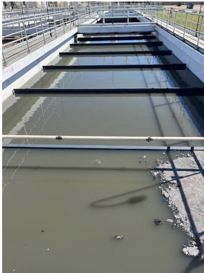
Figure 6: Rehabilitated PST No. 5. in service (USIBWC 04/17/2024)
