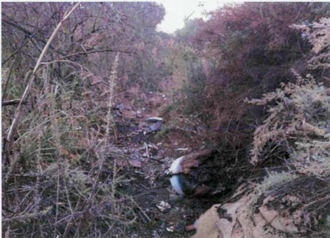
Photograph 4: Photo depicts downstream view of the drainage feature from the approximate midpoint of the proposed project.
