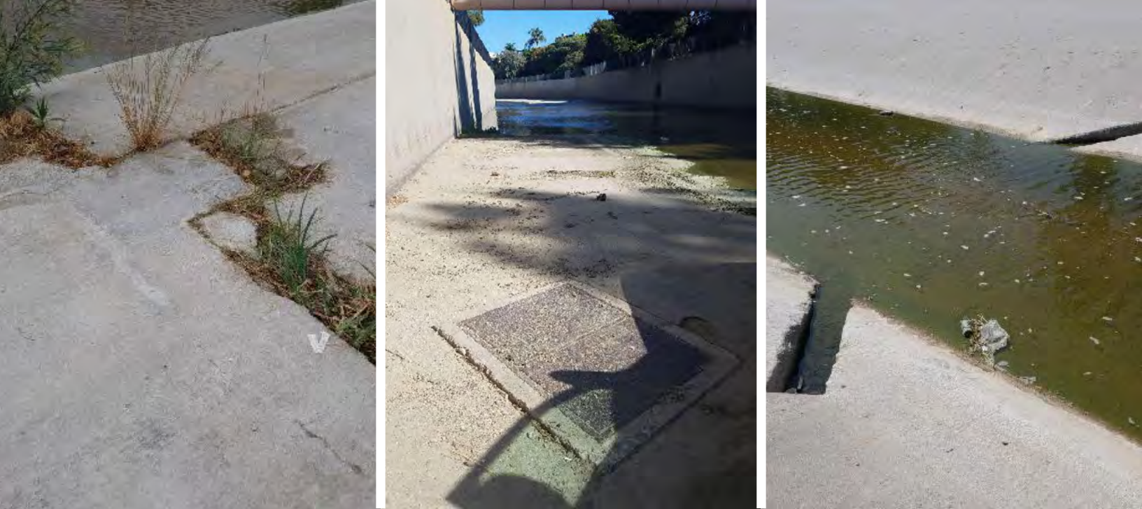
Figure 367. Channel lining, sub-drain hatch, and weep holes along the side of the LA River channel. Source: Geosyntec, 2018.
