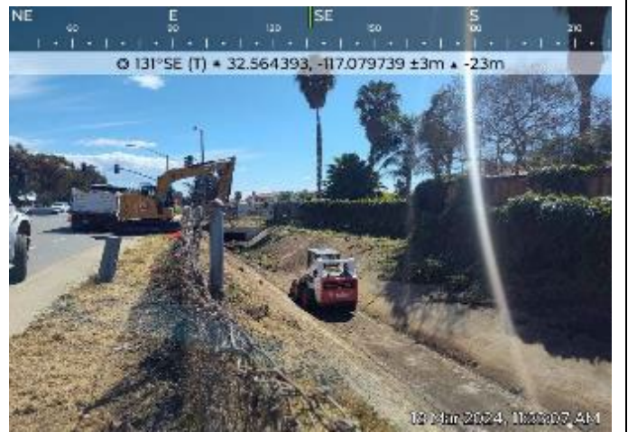
Tocayo 2 Post-Maintenance- Photo 2
