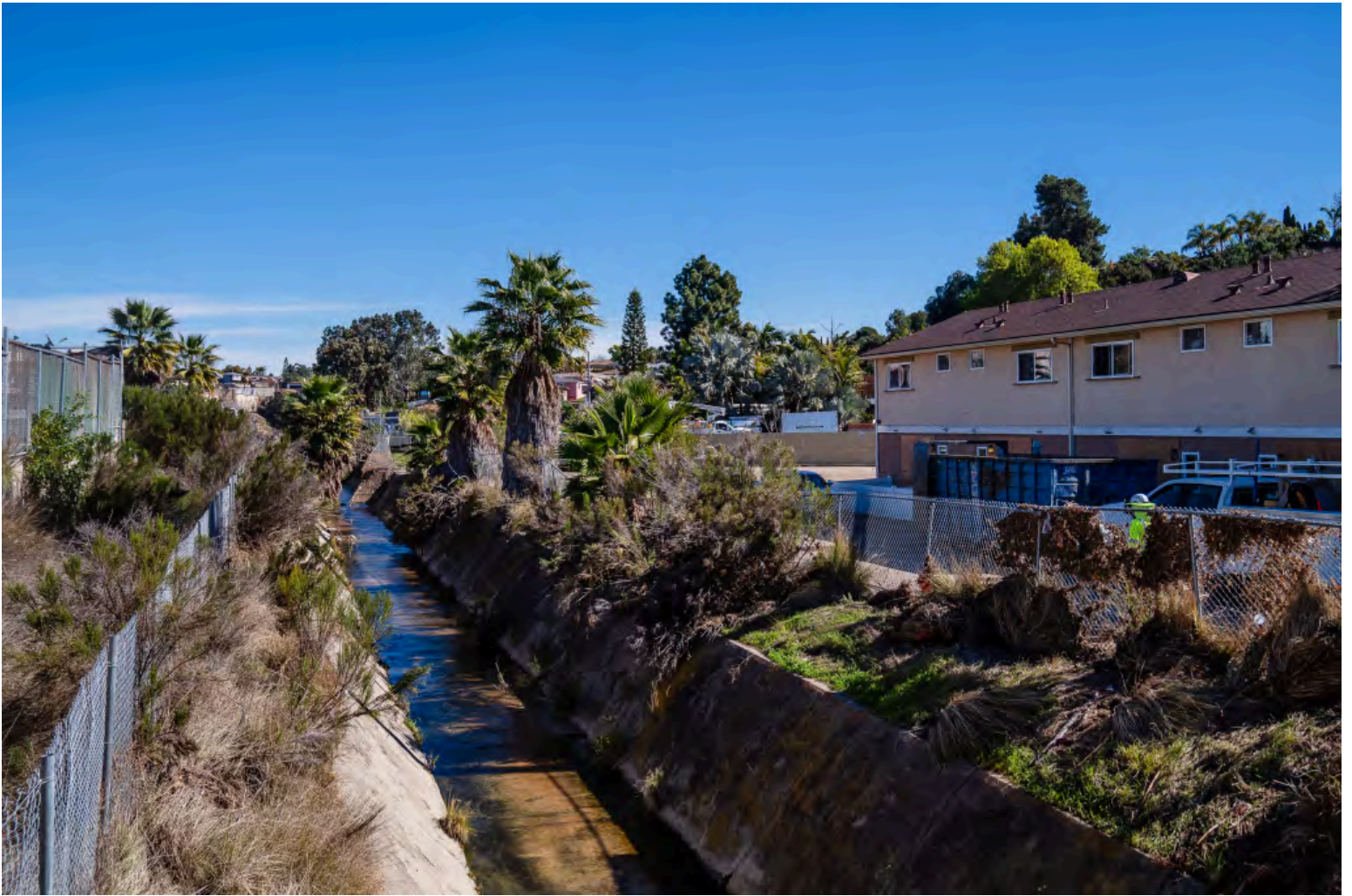
View of a channel alongside Village Green Apartments in Rolando that had already been cleaned out of debris and plant materials on Jan. 29, 2024. / Ariana Drehsler for Voice of San Diego
