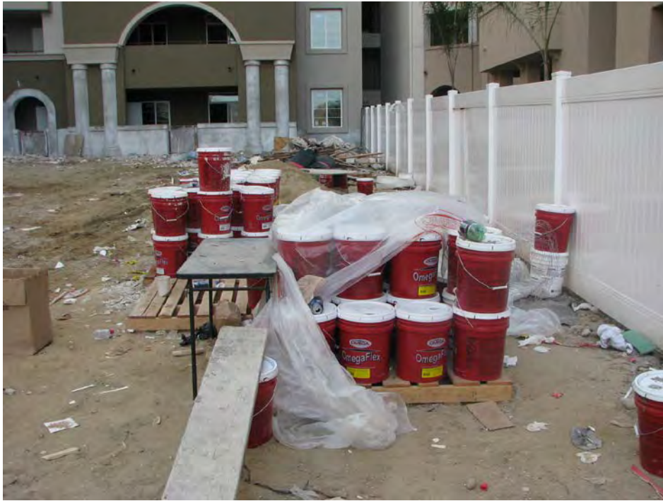
Figure 25. Improperly stored chemicals
