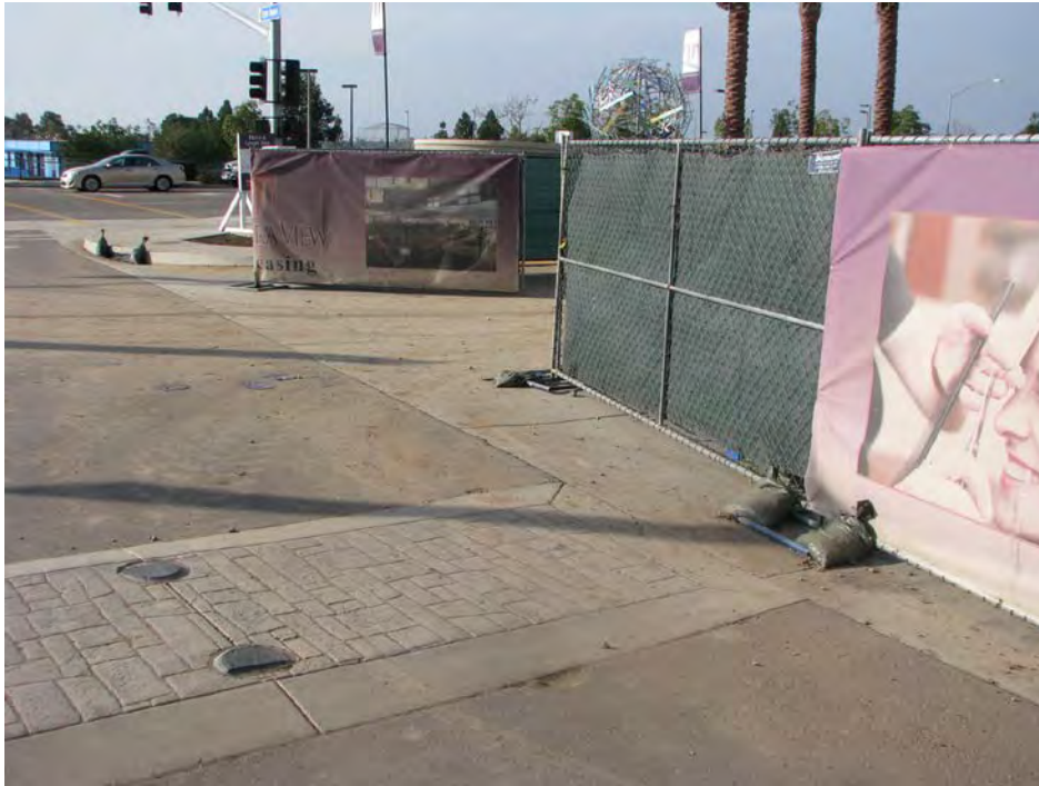
Figure 5. South-facing construction entrance; no BMPs; sediment tracking onto street
