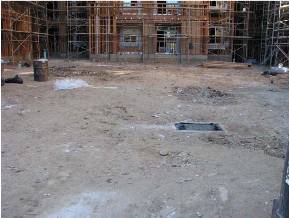
Figure 3. Site interior; inlet requires better protection
