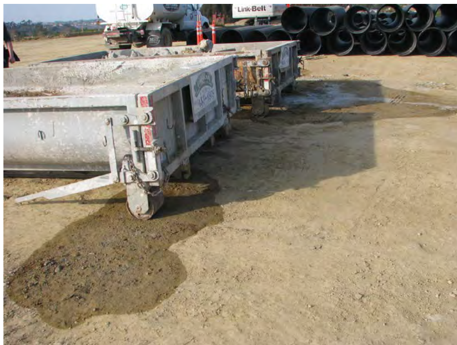
Figure 7. Leaking concrete washouts
