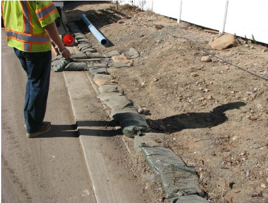
Figure 5. Site interior; linear sediment control BMPs not effective
