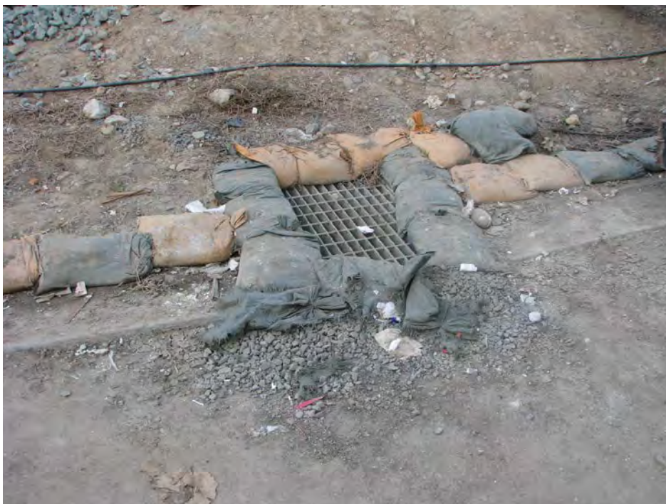
Figure 22. Broken gravel bags
