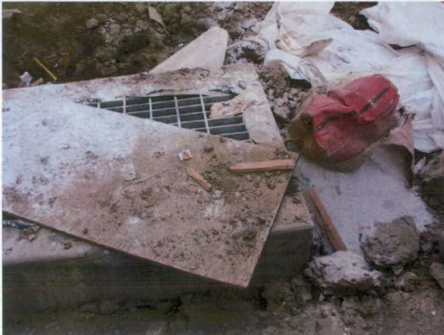
Figure 24. Storm drain littered with construction debris
