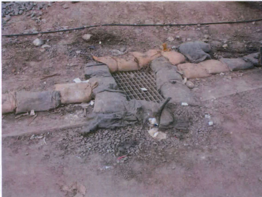
Figure 22. Broken gravel bags
