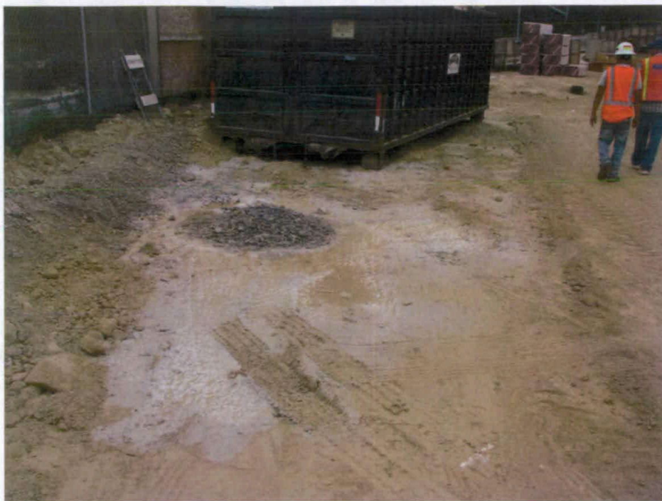
Figure 13. Concrete washout with no containment
