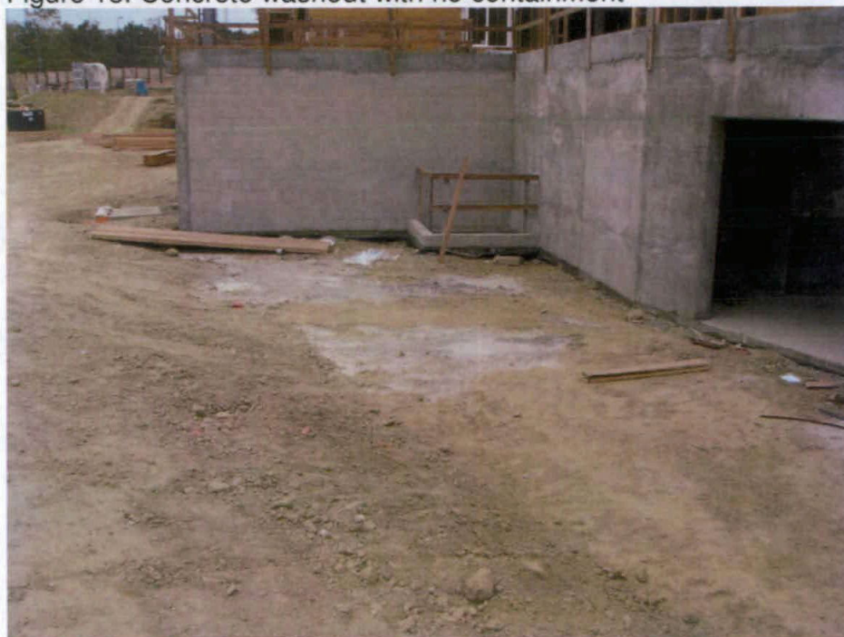
Figure 14. Concrete washout with no containment
