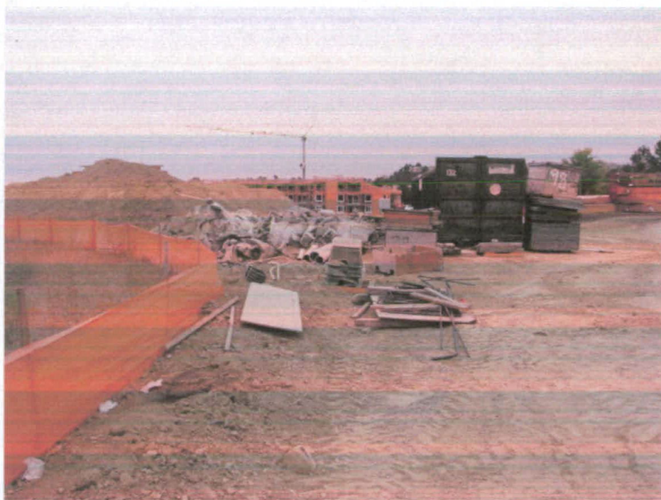
Figure 5. Site interior; construction debris
