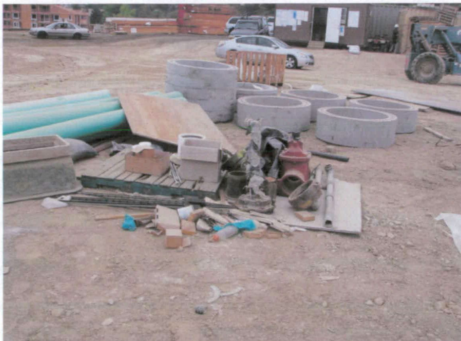
Figure 3. Site interior; construction debris
