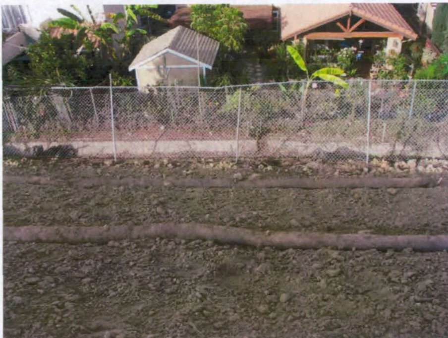
Figure 13. Damaged silt fence
