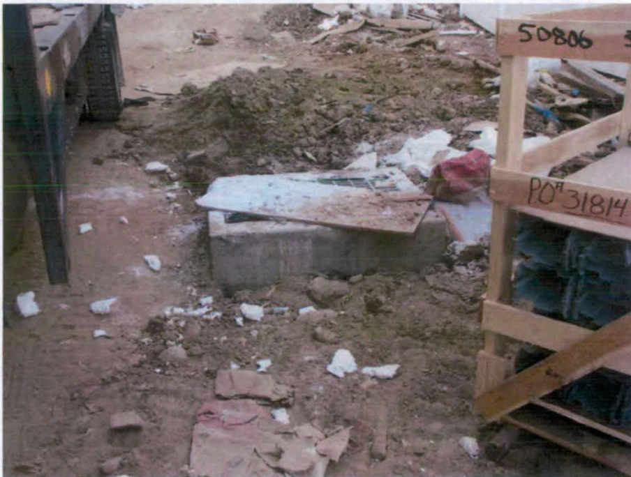
Figure 23. Storm drain littered with construction debris
