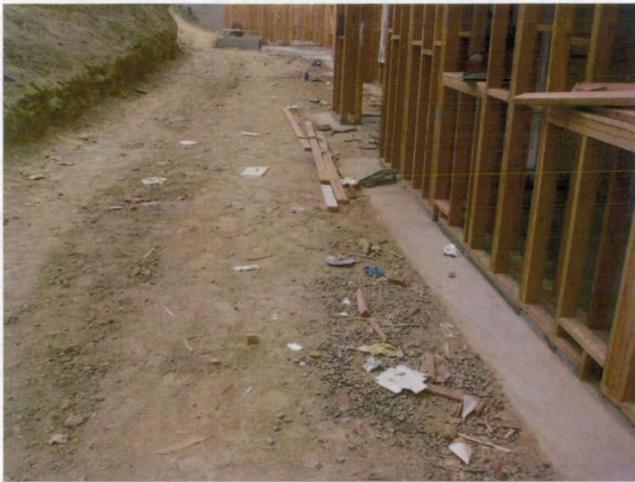
Figure 7. Site interior; trash
