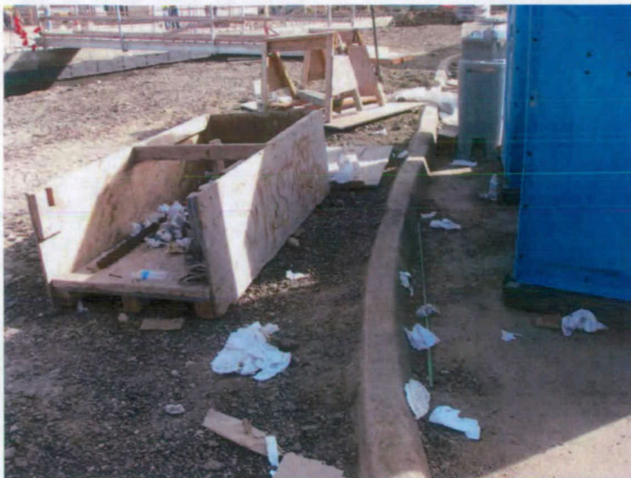
Figure 3. Site interior; trash
