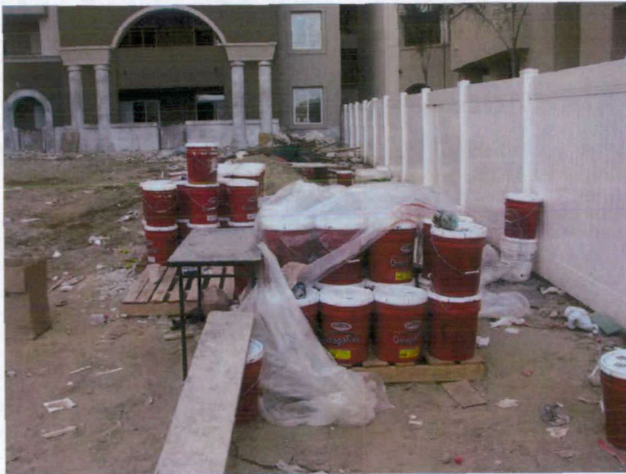
Figure 25. Improperly stored chemicals
