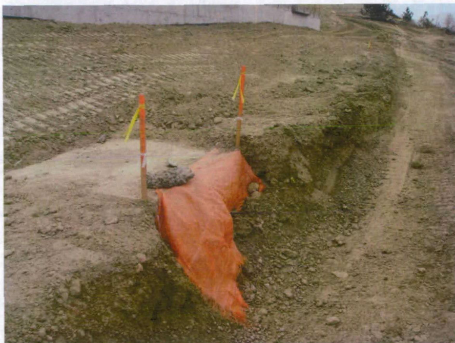
Figure 19. Live storm drain covered with permeable fabric
