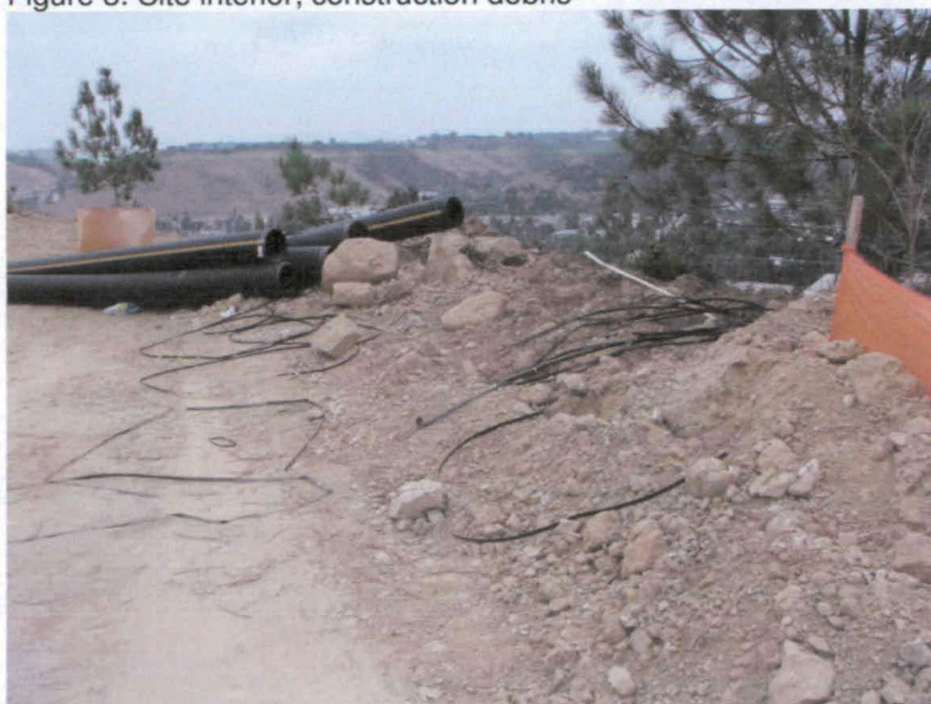
Figure 4. South west side; construction debris
