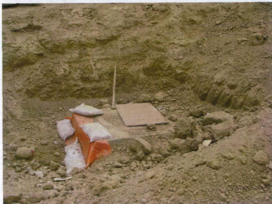
Figure 20. Live storm drain covered with permeable fabric
