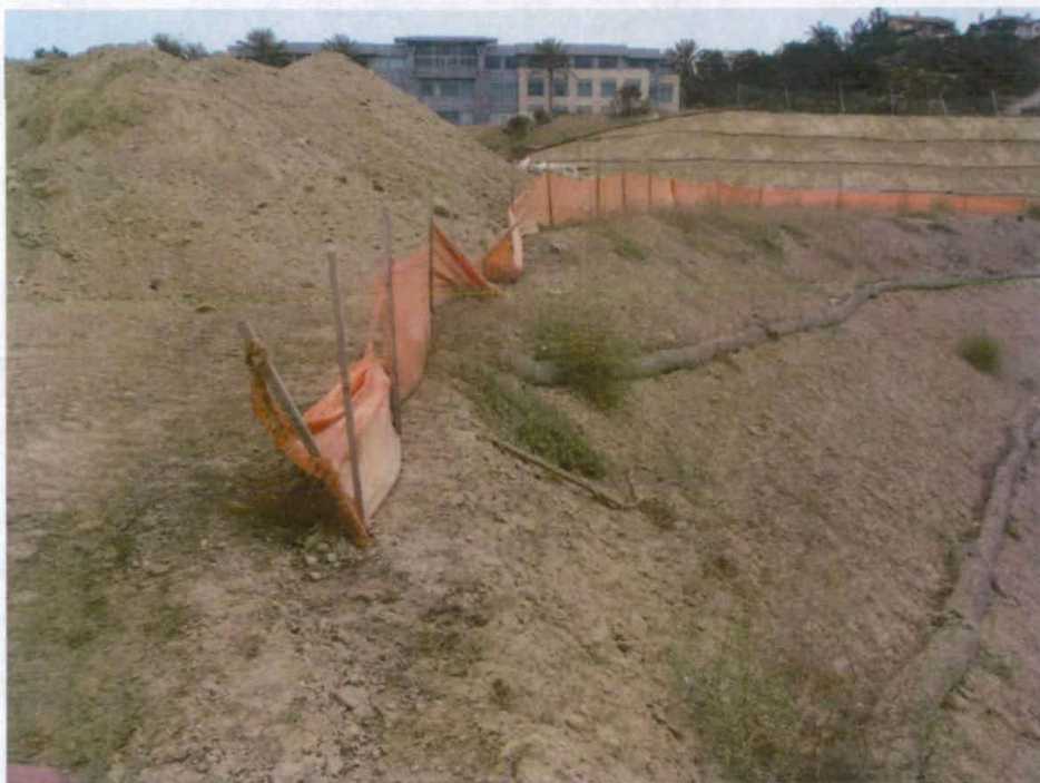
Figure 9. Sediment stockpile with broken silt fence
