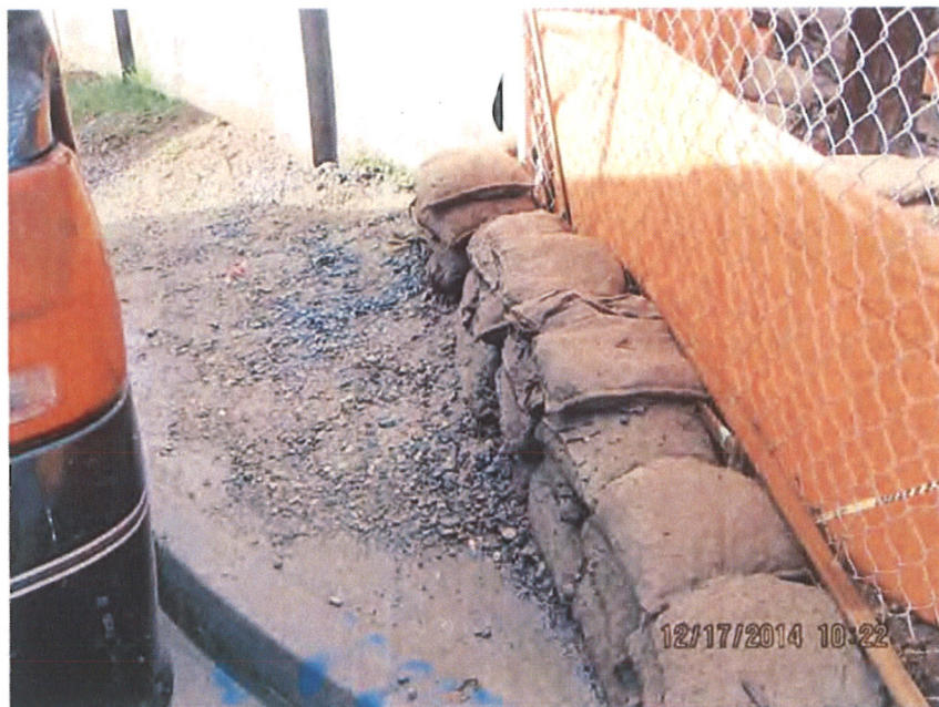
Photo 2. Evidence of sediment discharge at Akins entrance/exit
