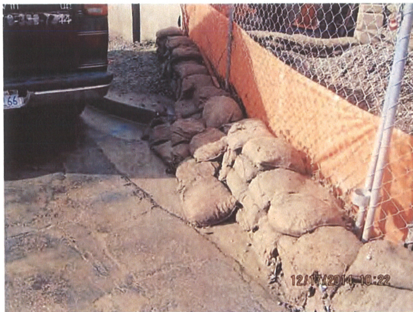
Photo 1. Evidence of sediment discharge at Akins entrance/exit
