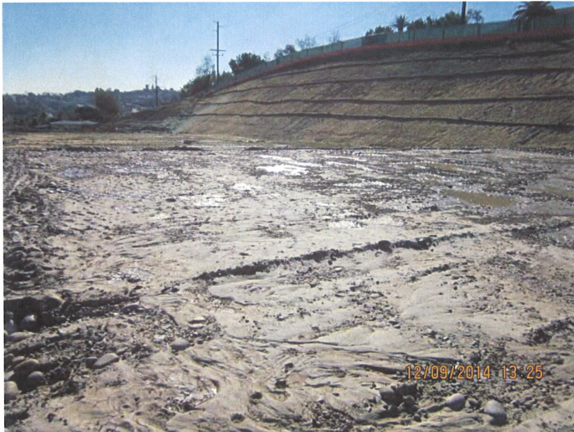
Photo 1. Lot lacking erosion control BMPs
