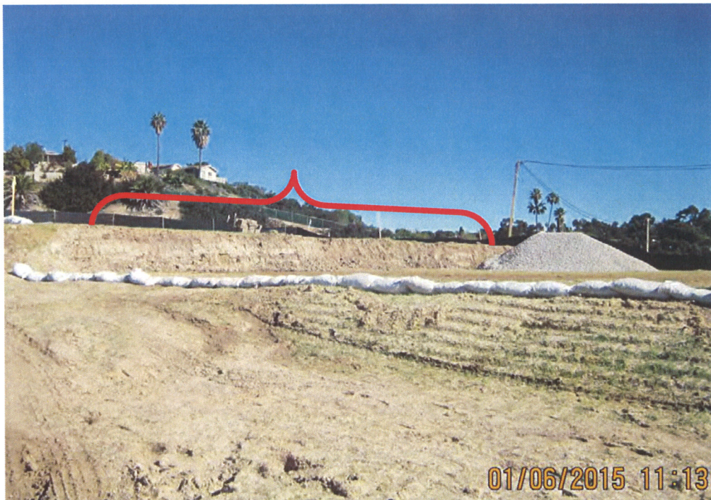
Photo 5. Sidewall without adequate erosion control
