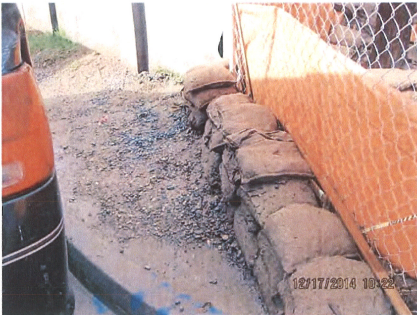
Photo 2. Evidence of sediment discharge at Akins entrance/exit
