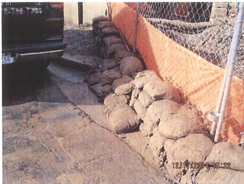
Photo 1. Evidence of sediment discharge at Akins entrance/exit
