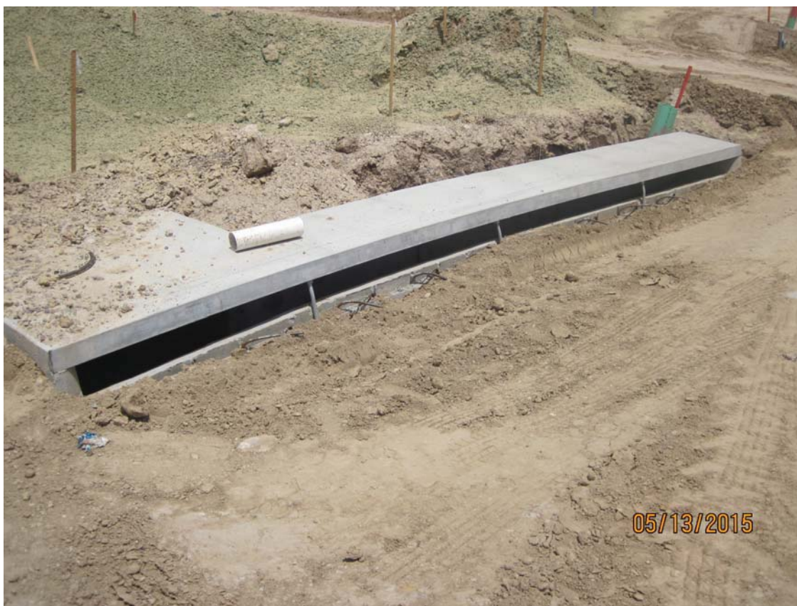
Figure 11. Failure to protect storm drain inlets. Photograph taken by Frank Melbourn, San Diego Water Board on May 13, 2015, displaying unprotected storm drain inlet. IMG_0295.jpg.
