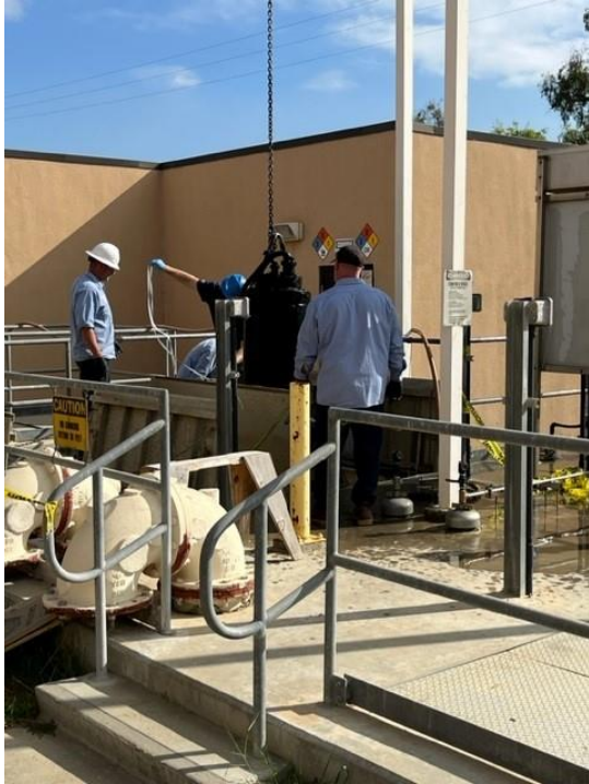
Figure 1: Pump Damaged by Tropical Cyclone Hilary
