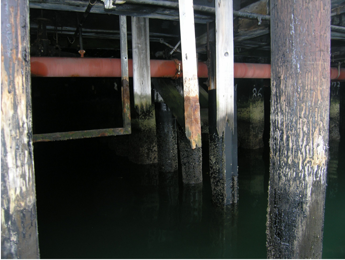
Figure 2. Many of the pilings at the Ninth Avenue Wharf are coated in creosote.
