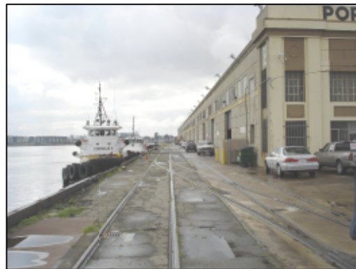
VIEW OF PIER SHOWING MULTIPLE OPEN DRAINS
