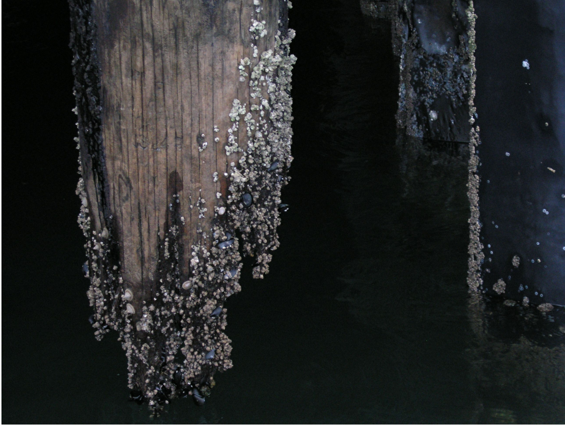
Figure 1. Broken pilings, hanging from the pier, were typical at the Ninth Avenue Wharf.
