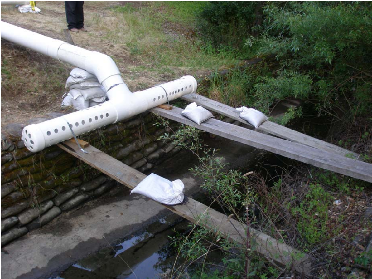
Figure 2: Discharge piping supported above a hardened section of channel
