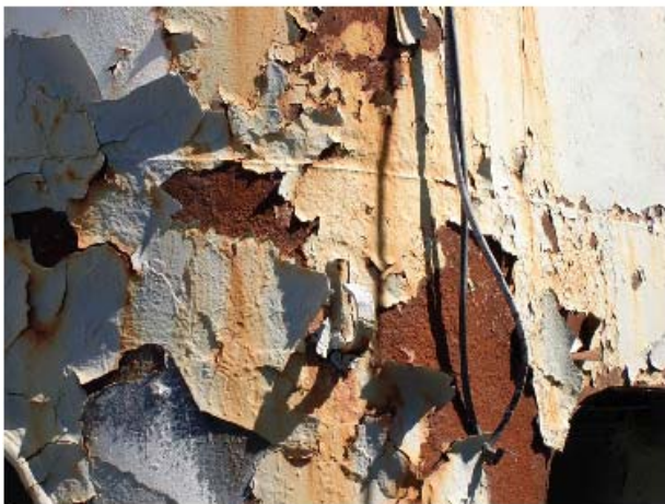
Photo #3 – Example of major paint exfoliation of an outboard surface
