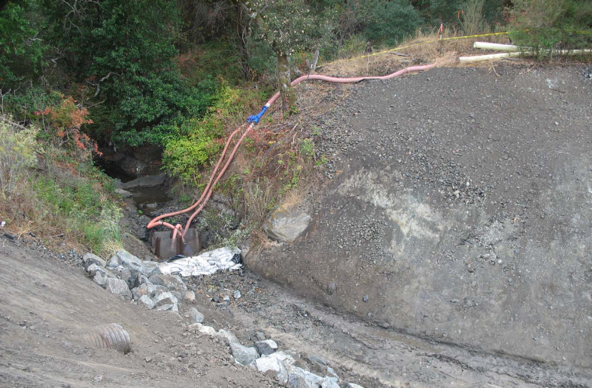
Dewatering Pumps and Cofferdam at Polhemus Crk Restoration Site – Upstream (South End) of Isolated Work Area 9-28-07 Photo #3 (HTK)
