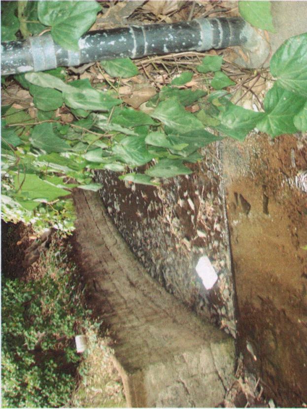
Sub optimal floodwall reach.
