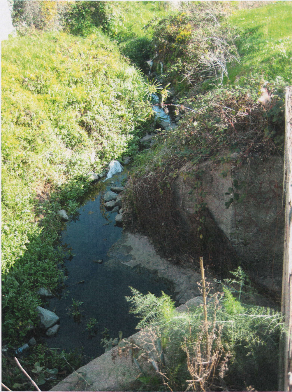
Baxter Creek reach west of San Pablo Ave, just prior to entering cement channel
