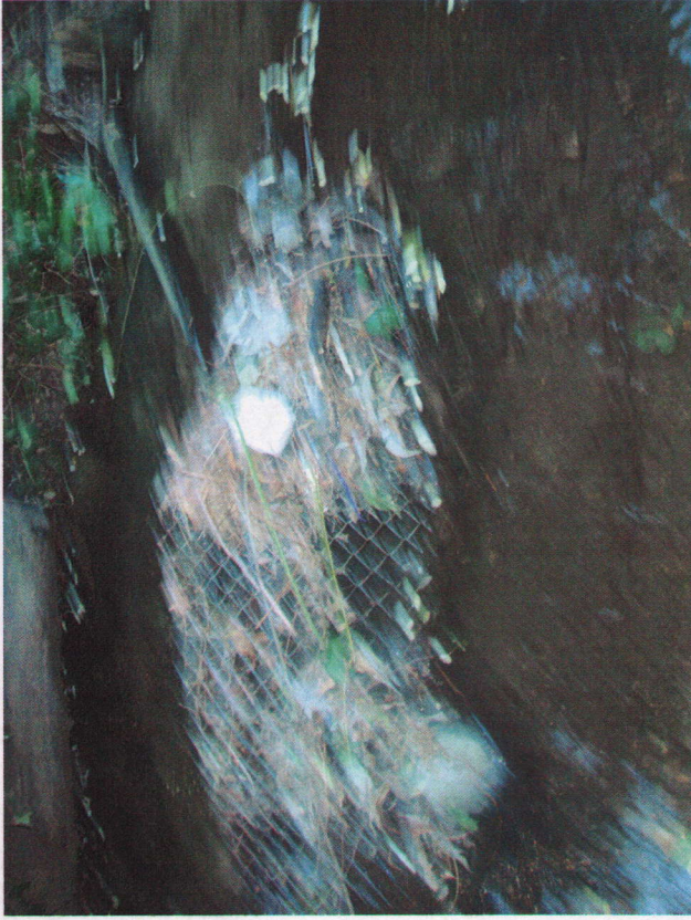
Sub optimal conditions with accumulations at collapsed gabbion.
