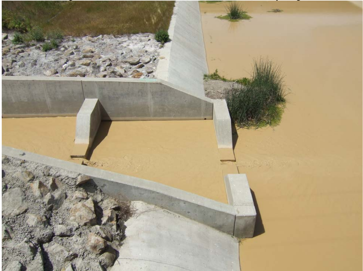
Photo of Receiving Water at Fish Ladder Structure Downstream of Facility, August 29, 2007
