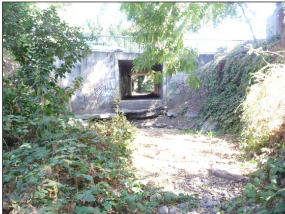
(1) Looking upstream at the South Terrace Road culvert crossing. Note the significant drop in bed elevation at the culvert and steep streambanks bounding the channel (September 2010).
