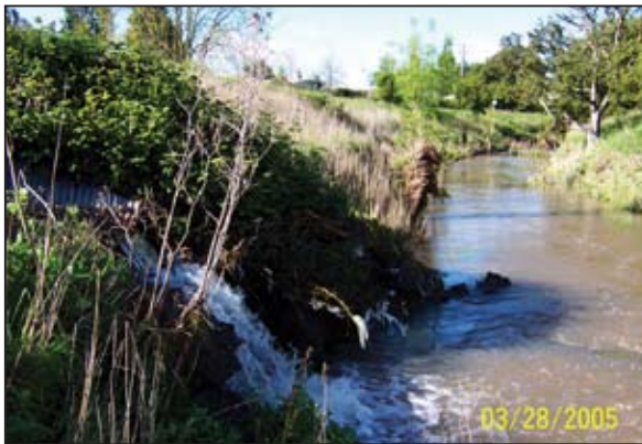
Photo 1. Example of a Culvert Failure.
