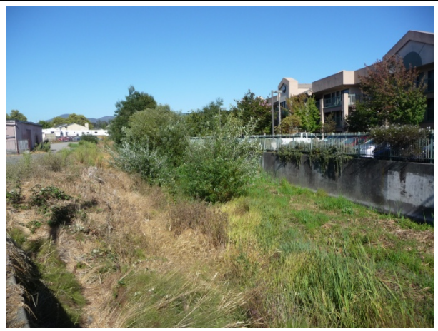
(4) Looking upstream from Soscol Ave crossing. Abundant sediment collects in a large and well developed mid channel bar (sediment wedge). Vegetation grows on deposited sediment, debris is caught on bar too. September 22, 2010).
