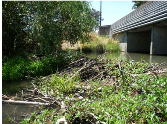
(2) The first beaver dam located approximately 600 ft downstream of Trower Ave. Dam pools water upstream as seen in Photo 1 (July 8, 2010).
