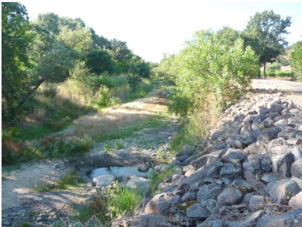
(3) Looking upstream at the riprap section where the channel turns towards the west. Erosion-resistant riprap sloughed into the channel has resulted in some local bed scour and pooling (August 4, 2010).
