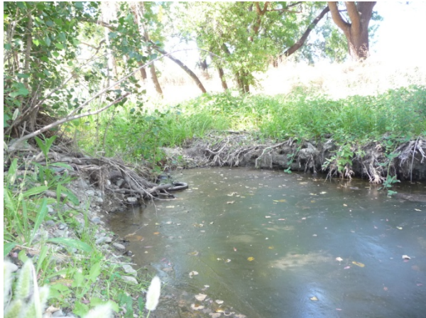
(3) 2-3 ft deep headcut is found midway through Reach 2. Tree roots provide bed stability at this location and the rate of headward migration appears slow ( Looking upstream near the middle portion of the reach, August 4, 2010 ).
