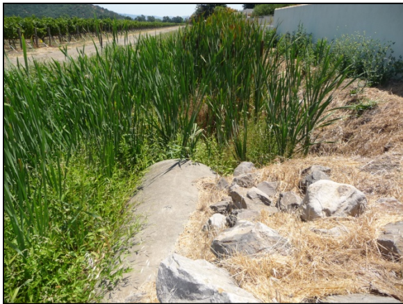
(1) Looking downstream from Finnell Road. Dense emergent vegetation occludes the culvert at this crossing (August 4, 2010).
