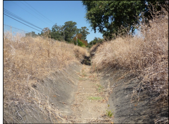
(2) Looking downstream from the mid-point of the Solano Ditch. The channel bottom and low banks are lined with concrete. The upper banks are formed in native soils. Vegetation on the upper banks consists of non-native herbaceous species (August 4, 2010).
