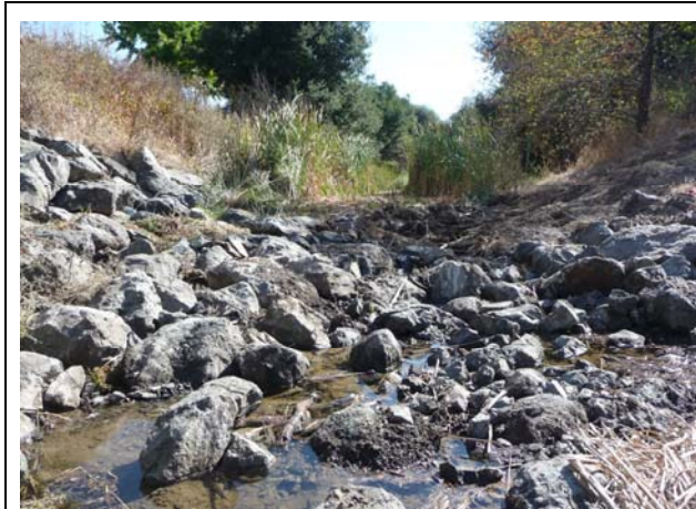
(3) Looking upstream near Highway 29 crossing. Recent riprap was placed along banks and channel bed. Channel bed and riprap crossing create depositional area upstream where sediment accumulates and cattails grow (September 22, 2010).
