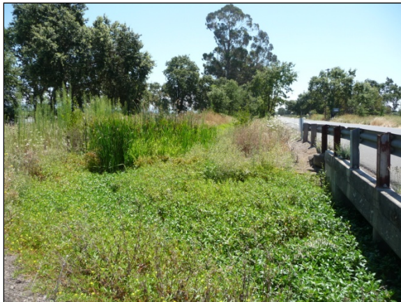
(1) Looking downstream from upstream end of the NYC. Two concrete box culverts pass flows from the main upstream tributary into the NYC. Note the dense aquatic and emergent vegetation in the channel (August 4, 2010).
