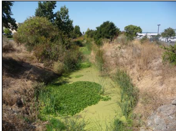
(1) Looking downstream (west) from the bridge at North Kelly Road (September 2010). Stagnant water and poor water quality observed.
