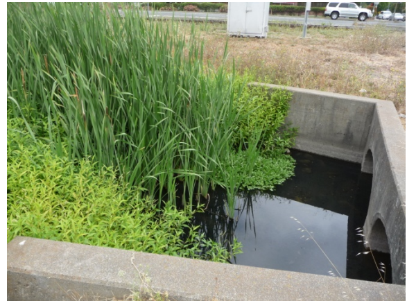
(2) Culvert outlet at upstream end of the SSC. Water clarity at this location was good (August 2010). Note emergent vegetation growing immediately downstream of outfall.
