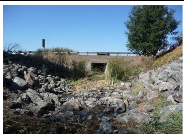
(4) Recent bank stabilization work performed by District included riprap placement upstream of the Highway 29 culvert crossing (view is looking downstream, September 22, 2010).
