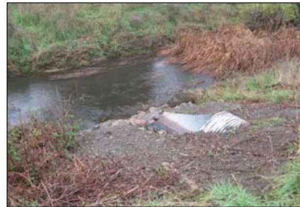
Photo 2. Same site as Photo 1 after bank repair using minimum necessary rock rip-rap.
