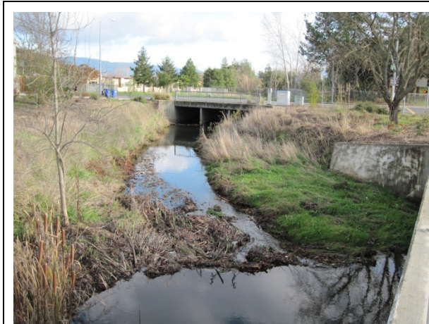
(5) Sediment accumulation along the south bank (right side of photo) between Jefferson St. and Trower Ave. (December 2009).
