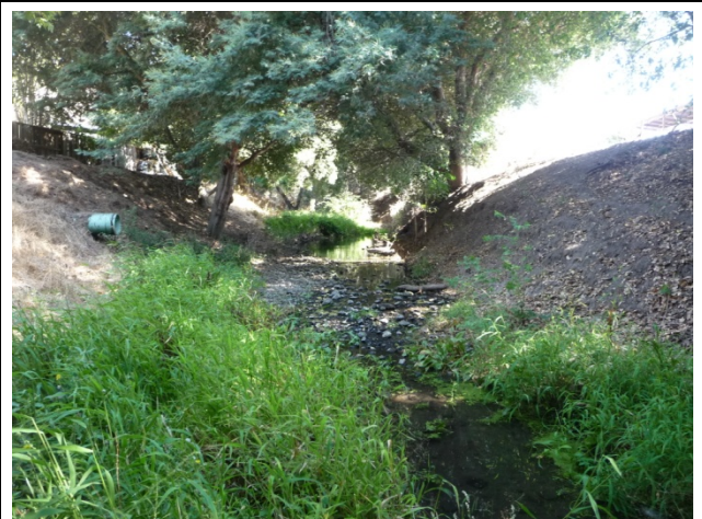
(4) Typical conditions in the lower portion of the reach (Looking upstream, September 22, 2010).
