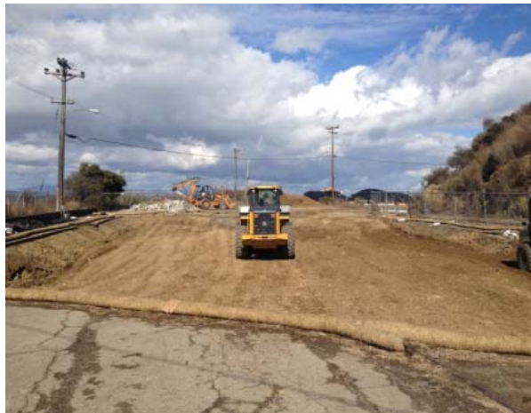
Photo 1b. Excavation at Vopak was completed and backfilled with clean material, prior to repaving with asphalt (looking north).
