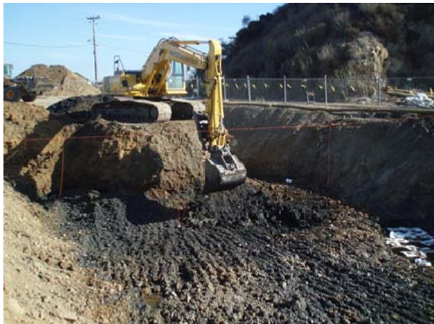
Photo 1a. Excavation around one of Vopak's unknown USTs that had caused extensive staining (looking northeast), and absorbent pads on groundwater surface soaking up oily sheen (east side of excavation).
