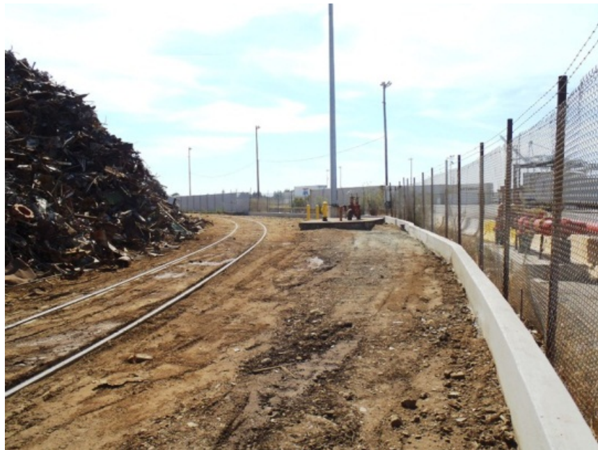
New extension of concrete containment wall along southwestern facility boundary. Over 600 lineal feet of new containment installed. Project completed August 24, 2012.
