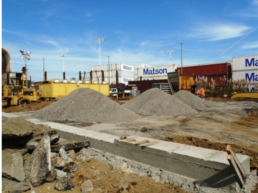
Grading, base preparation and footing construction underway to install additional tent structure to expand covered maintenance area. Expected project completion – October 31, 2012.
