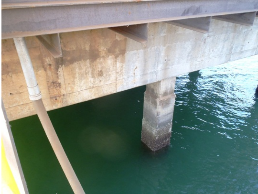
Demonstration of dock cleanup effectiveness. Dock face in right portion of photo has been cleaned. Dock cleanup activities completed September 6-14, 2012.
