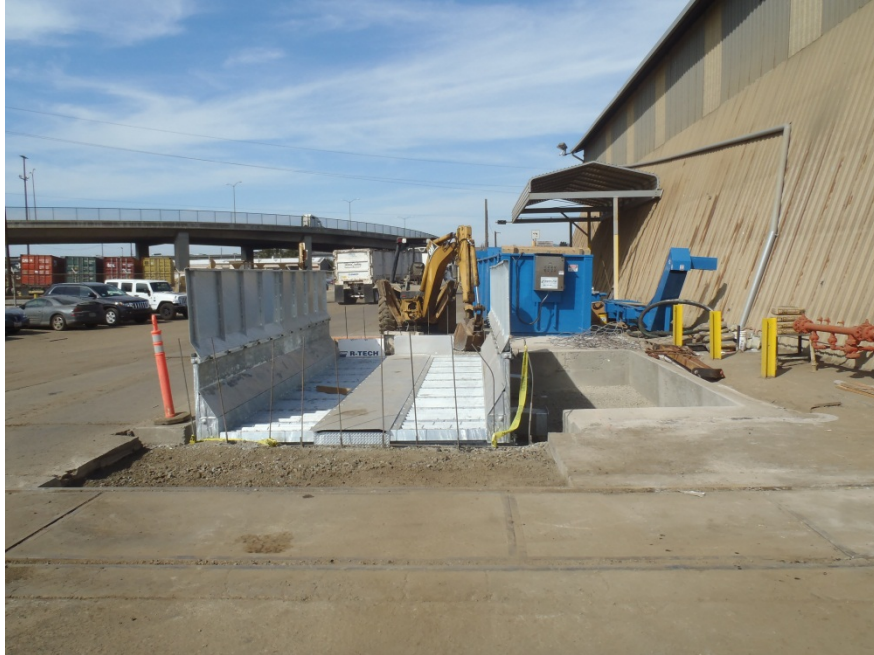
Construction project underway to install commercial wheel washing station at facility exit. Expected project completion – October 1, 2012.
