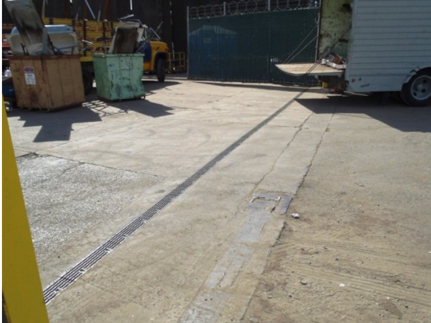
New strip drain to prevent off-site flow of stormwater at retail non-ferrous department entrance. Project completed – May 2012.
