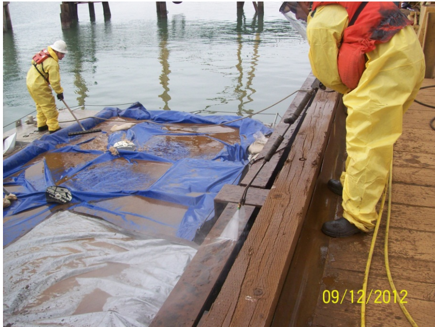
Dock cleaning activities. All wash water was captured by containment barge, profiled and disposed off-site. Dock cleanup activities completed September 6-14, 2012.
