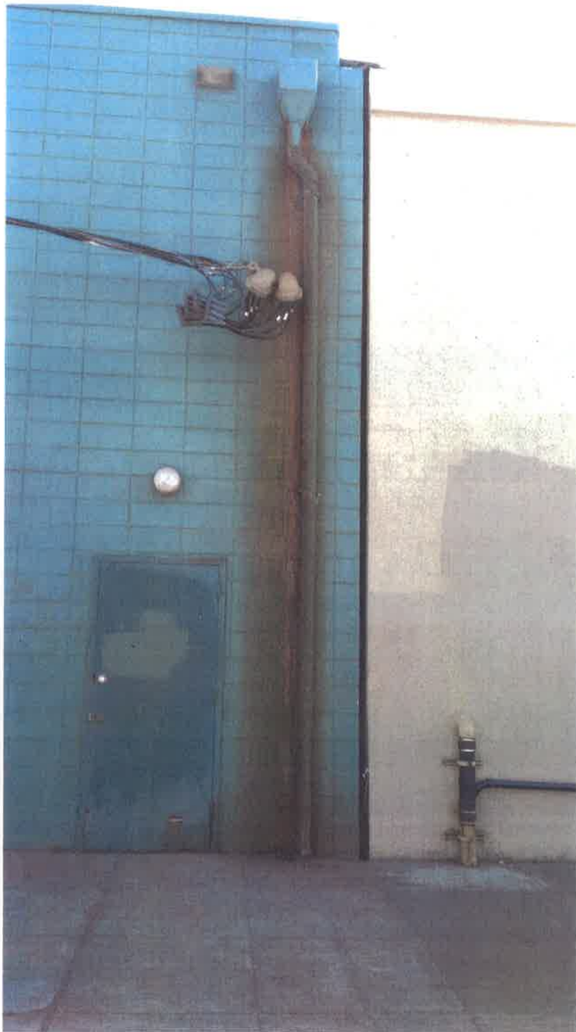
Photograph a – Discoloration of green paint on and around roof drain pipe from E – D Coat, Inc. facility located at 715 4th Street, Oakland, California 94607. Photograph taken by David Williams on June 3, 2013, at 5:15 p.m., looking south at the front of the facility from 4 th Street.
