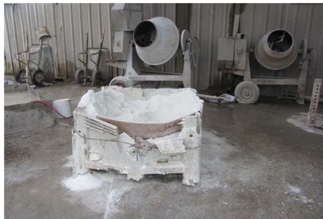
Photo P: Aggregate mixing with Storm Water
