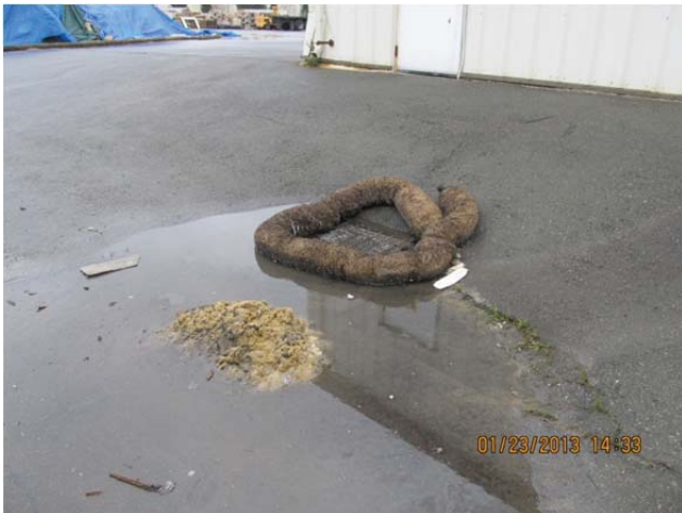
Photo D: Storm Water Drop Inlet w/ Accumulated Sand
