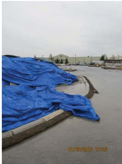
Photo S: Unsecured Cover in place over Concrete-related Materials
