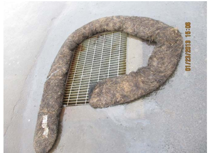
Photo T: Unmaintained Fiber Roll and Oily Sheen
